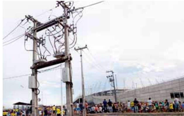
NOJA Power's OSM auto reclosers used to protect Castelão stadium's electricity distribution feeders.
