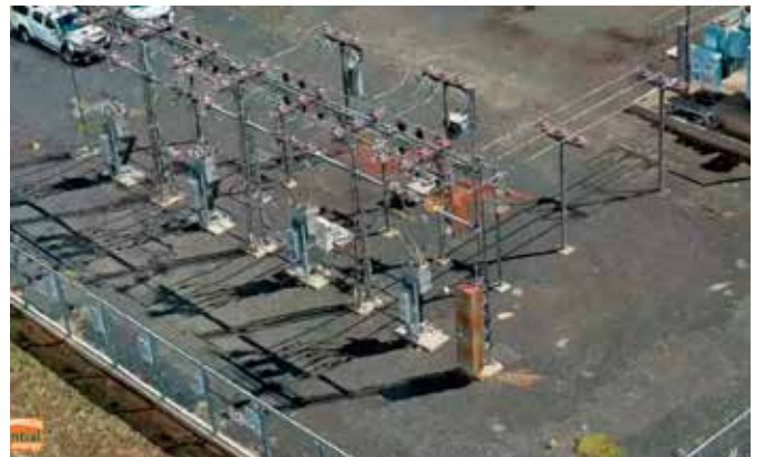
Digital reality model of the Brewarrina substation. Image courtesy of Essential Energy.
