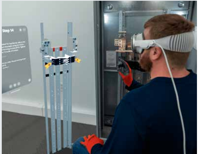
A man wearing an Apple Vision Pro next to a Siemens P5 power panel. He is looking at a digital overlay of BILT immersive instructions including a 3D rendering of the panel and a text window.
