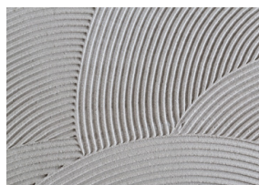
NO Incorrect application
