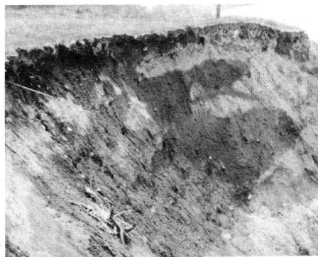
Figure 11. Dark, moist bands indicate groundwater seep zones.
