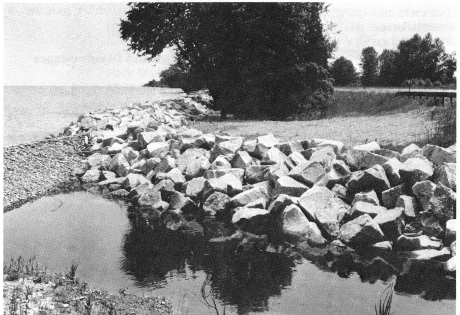
Figure 22. This rock rip rap revetment contains a filter layer, armor stone, and toe protection to prevent undercutting by scour.
