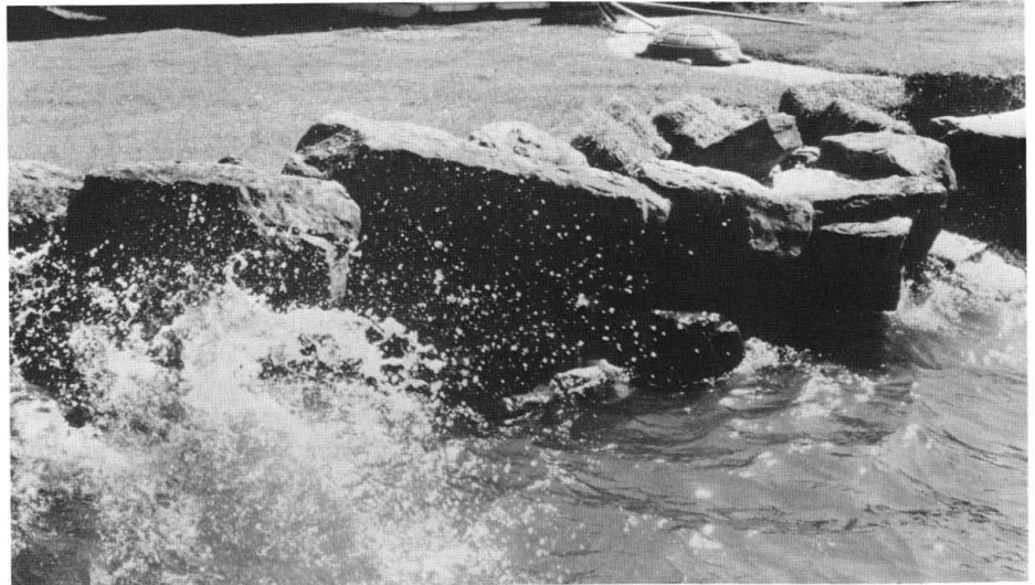
Figure 3. Overtopping can easily lead to structure failure if measures are not taken to prevent the land behind from being washed away.
