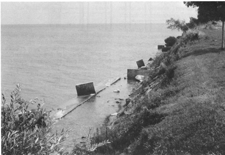
Figure 8. Lack of tie backs and deadmen led to this bulkhead's failure.
