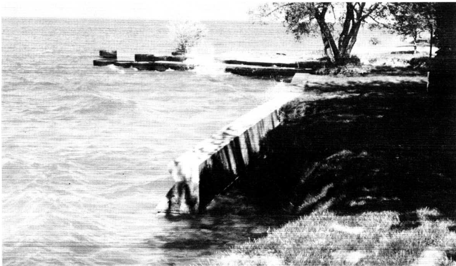
Figure 6. Without wingwalls or returns, flanking can lead to a structure's premature failure.
