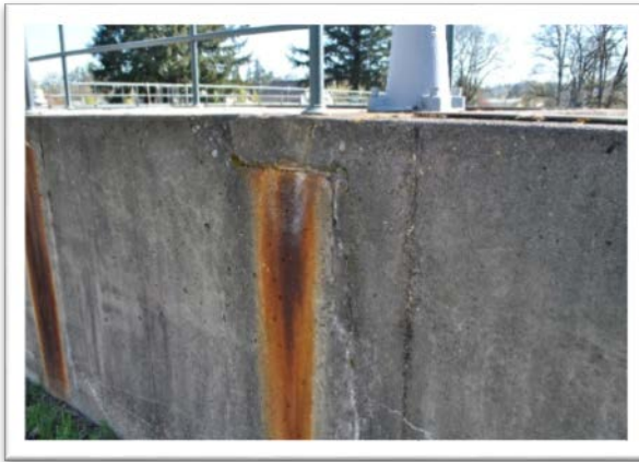
Figure 6-9. Sedimentation Basins Concrete
