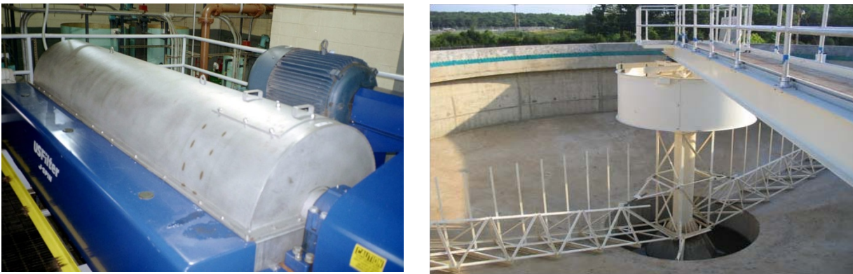
Figure 2-14. Example Photographs of a Centrifuge Dewatering Unit (left) and an Empty Gravity Thickener (right)
