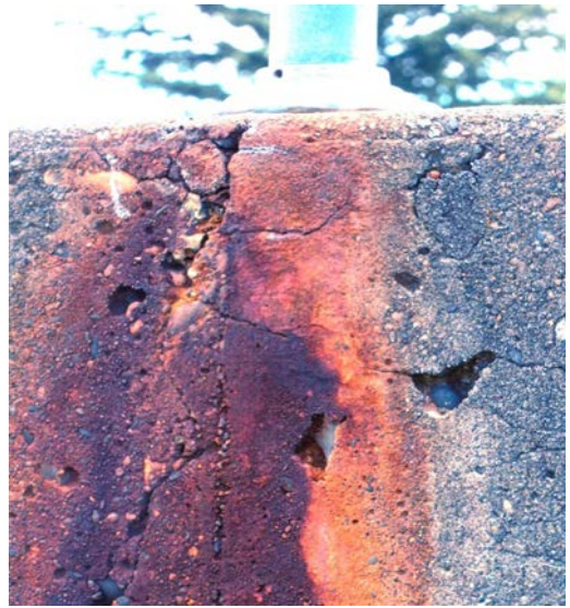
Figure 4-4. Guardrail Anchorage Corrosion
