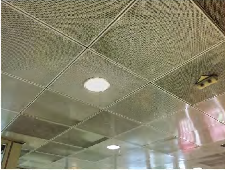
These painted metal ceiling panels can be rejuvenated by wiping with a degreasing cleaning agent. However, the non-woven acoustic fabric behind the perforations may have to be replaced since grime attached to the fabric is more difficult to remove and may also interfere with noise reduction.
