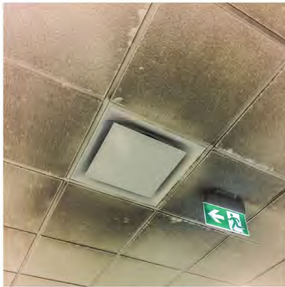
Dust, soot, grease, and other schmutz can accumulate around air diffusers due to the Coand effect. Panels with textures and tegular edges provide additional surface area to trap contaminants and make cleaning more challenging.
