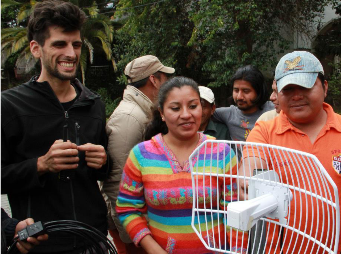
Figure 6.2: Participants learning how to install a Wi-Fi network in the fifth module of the first edition of Techio Comunitario , developed in Guelatao de Juárez, Oaxaca
