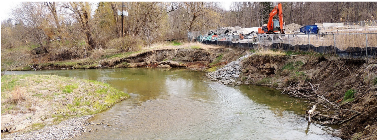
Figure 4.5: Stream bank erosion.
