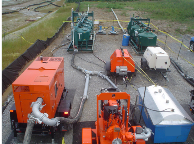
Figure B2-26: Active water treatment system for construction site runoff
