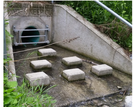
Figure B1-12: Erosion blanket in an outlet area (top) and baffle blocks for energy dissipation (bottom)
