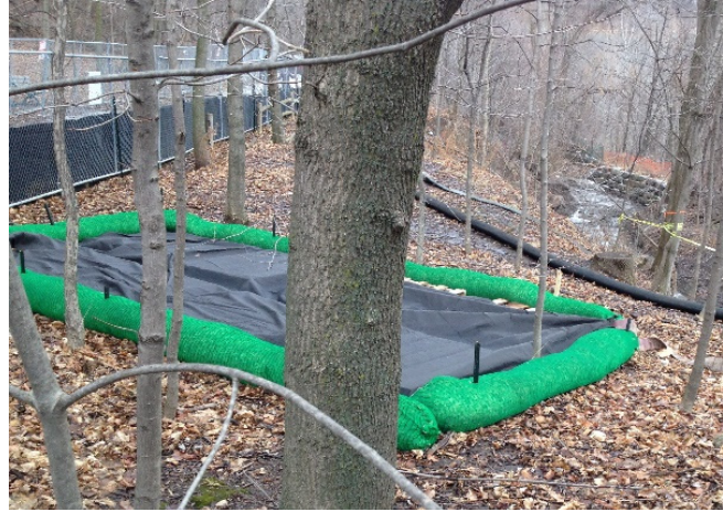
Figure B2-15: Sediment bag surrounded by filter sock
