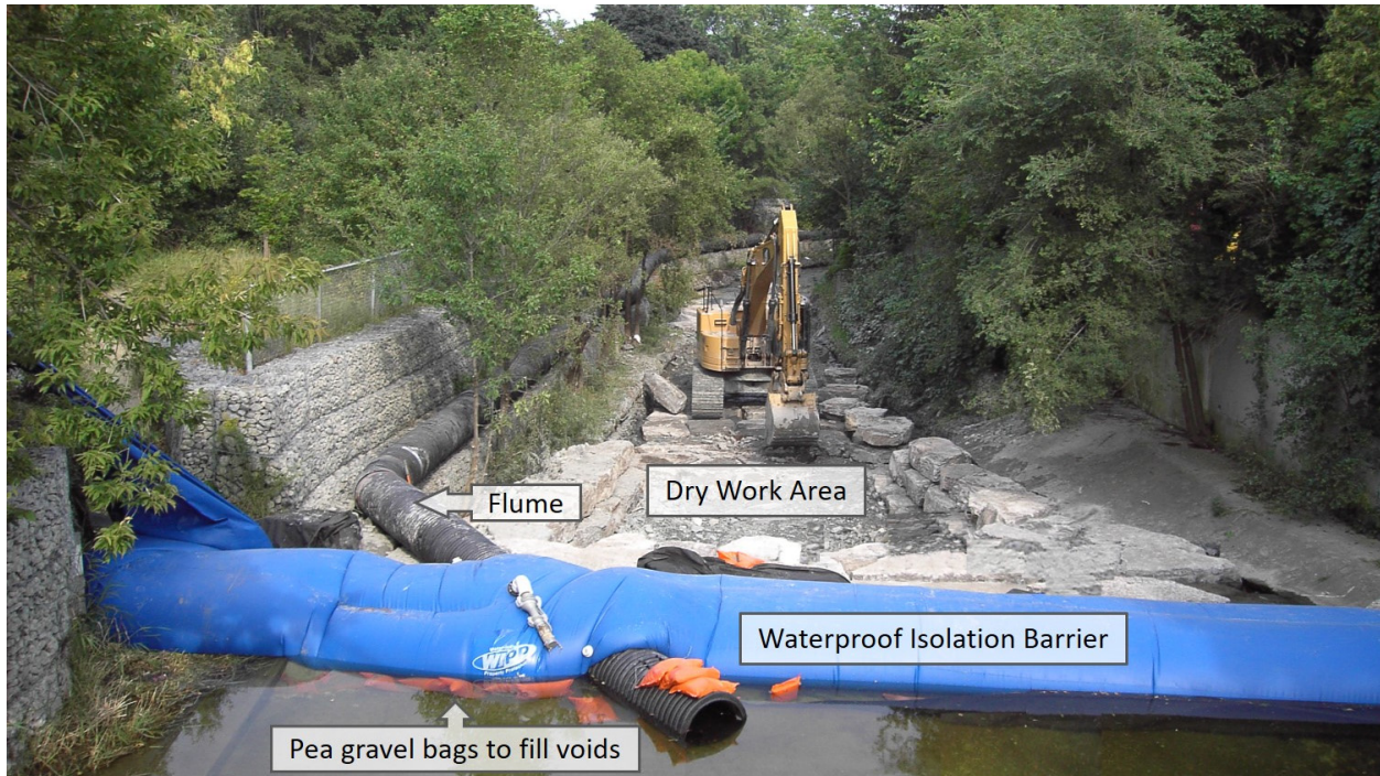
Figure C8: Application of a flume bypass to divert stream flows around a dry work area
