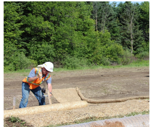
Figure B1-15: RECP installed on a slope and anchored in place at the top
