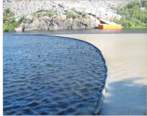
Figure 7.15: Turbidity curtain applied to isolate a work area when working in the wet
