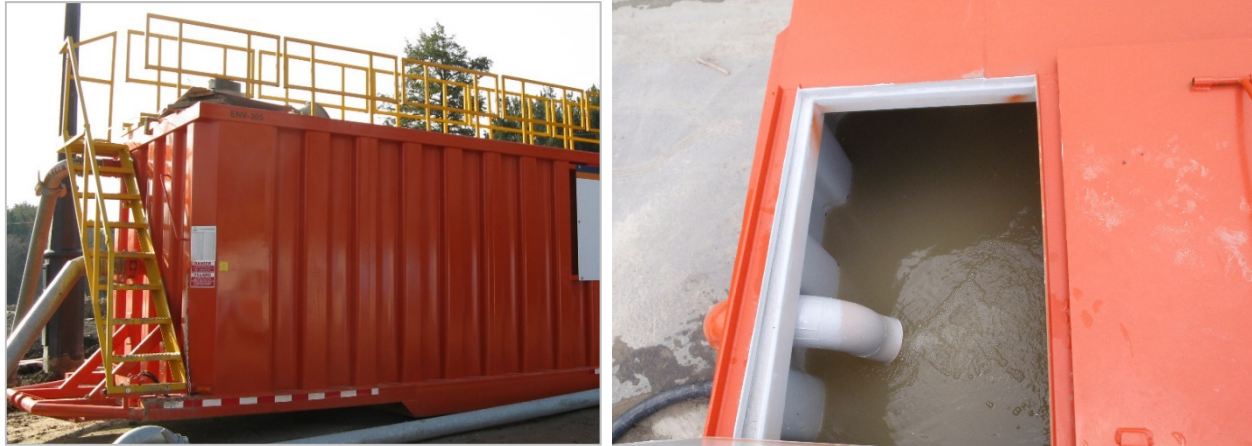
Figure B2-22: Weir tanks
