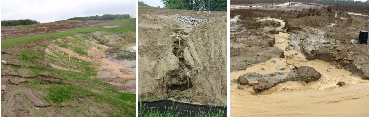
Figure 4.1: Rill (left) and gully (centre and right) erosion on construction sites.
