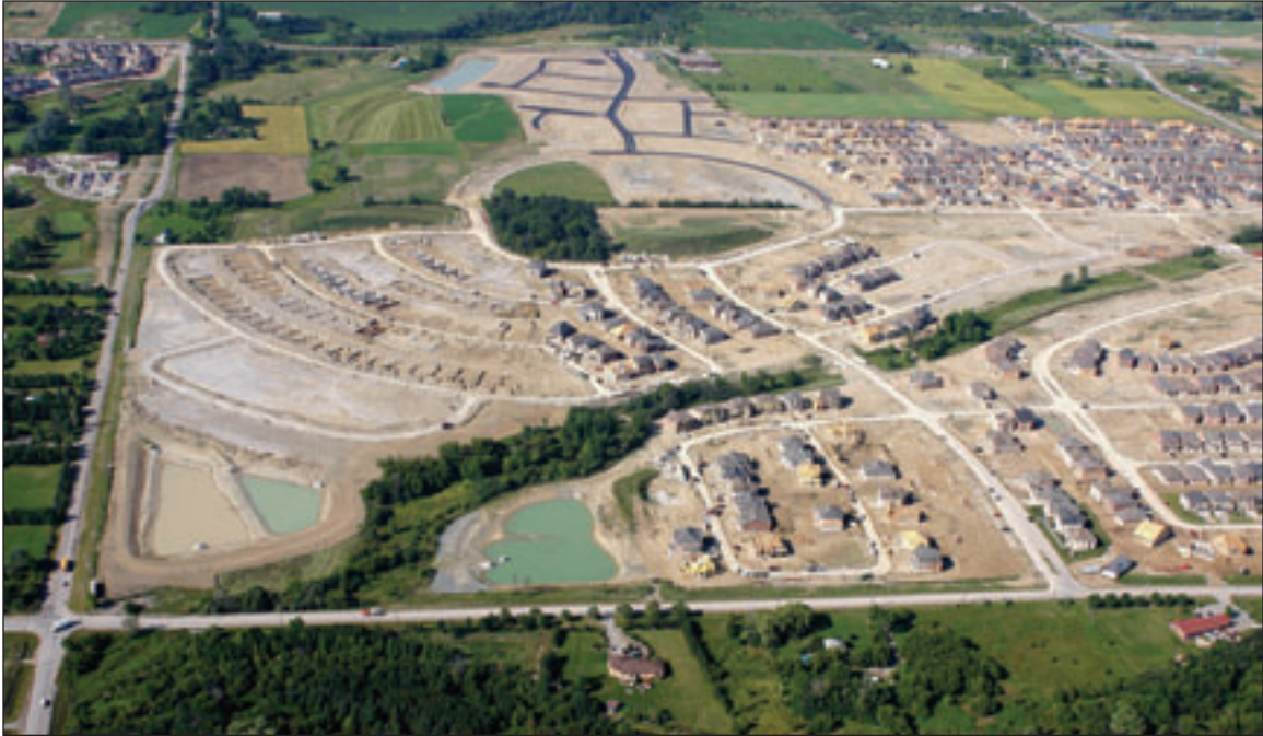
Construction site erosion and sediment controls and stormwater management ponds need careful installation and routine inspection and maintenance to function effectively. Photography by Lou Wise
