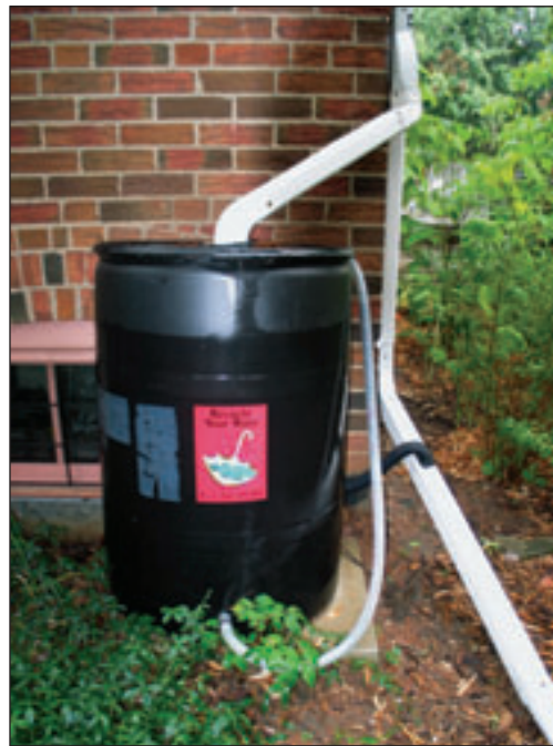
Rain water harvesting with a rain barrel (pictured here) or cistern helps to conserve water and achieve stormwater management objectives. Photography by Rose Hasner
