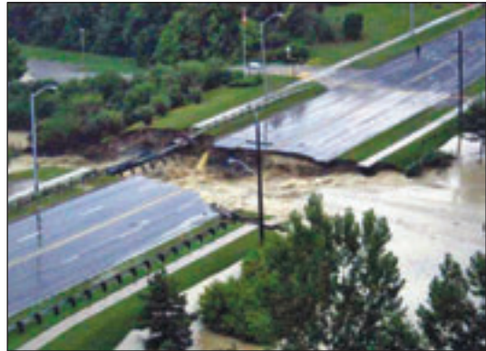
Finch Avenue being washed out by Black Creek during a major storm event on August 19, 2005. Photography by Tahir Rasul
