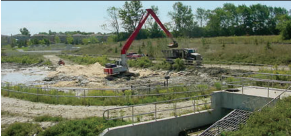
Stormwater management ponds need periodic maintenance to maintain performance. Photography by Town of Richmond Hill
