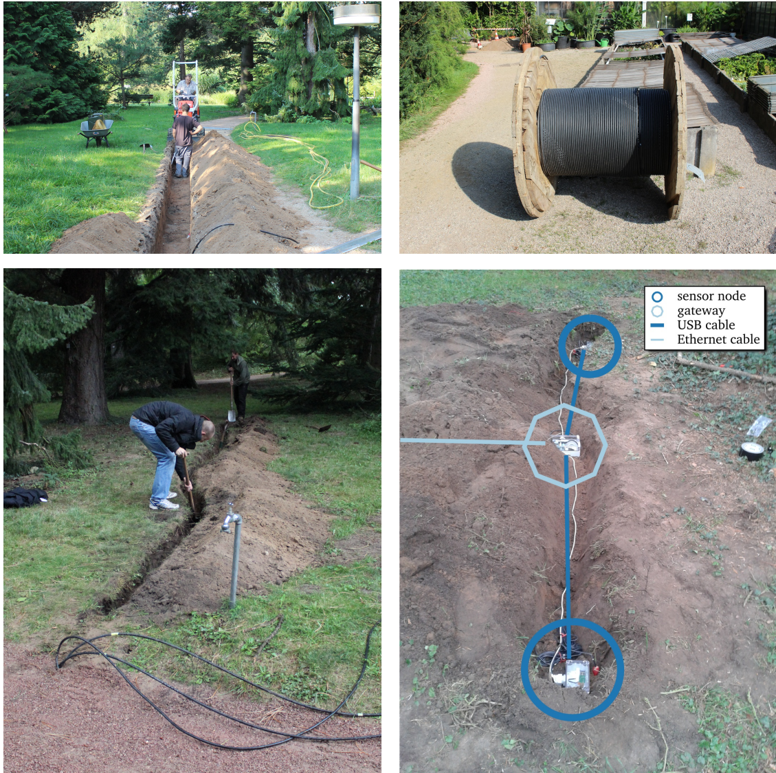
Figure 5.9.: Left to right, top to bottom: 1) digging work on main path for deployment of power and fiber-optic cables 2) at correct depth –minimum of 50cm–, 3) shoveling within the coniferetum to finally deploy 4) nodes and their enclosures
