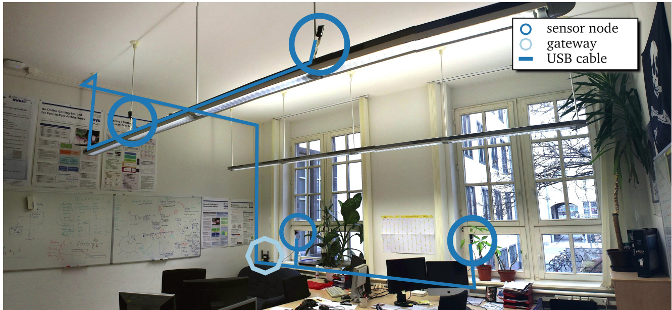
Figure 5.3.: An office in the Piloty building, with installed wireless sensors (circles) that are also attached to a gateway (octagon) for quick reprogramming.
