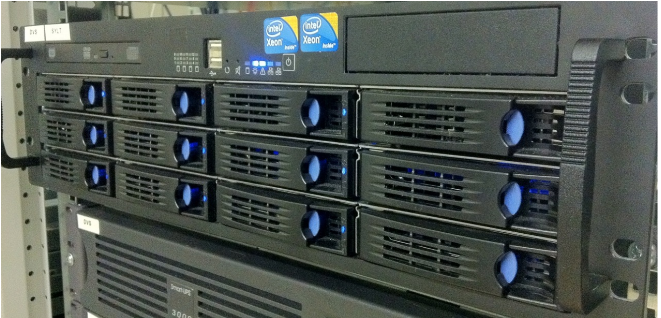
Figure 2.10: The Sylt Server testbed installed in the server rack.
