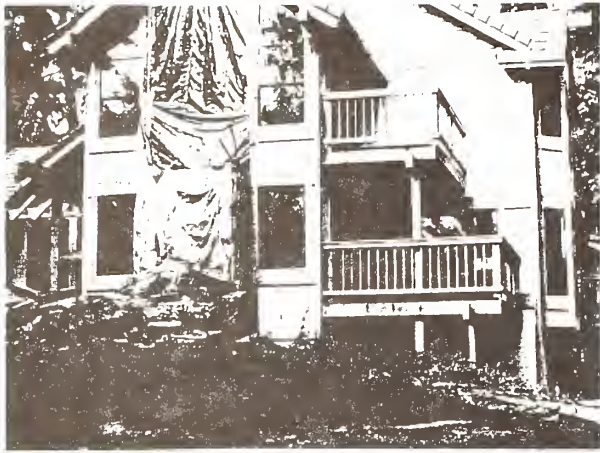
Figure 1. Two-story house with wood-framed daylight basement located about 100 feet from ground fissure in Santa Cruz Mountains. No apparent structural damage except collapsed masonry chimney.
