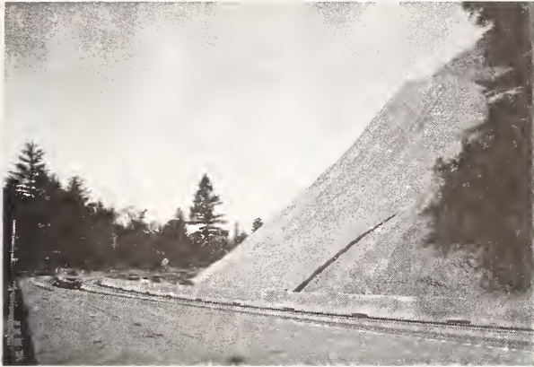
Photo. 1 Slope Failure along State Freeway No.17 (One of Largest Landslides caused by the Earthquake with Height \approx 20m and Length \approx 100m; It took one month to completely open this portion to the public traffic. This photo was taken in the end of November, 1989 after repair works finished.)
