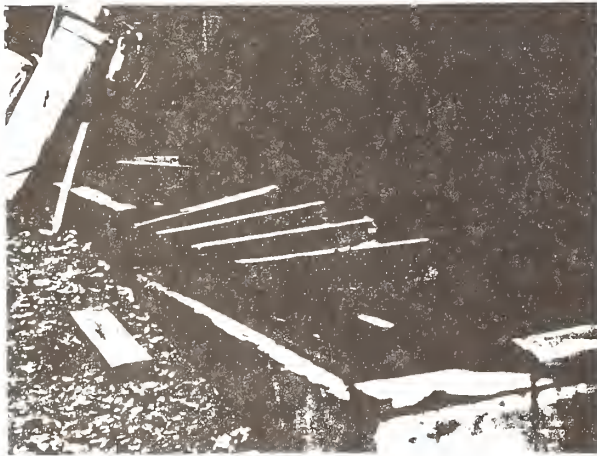
Figure 2. Collapsed cripple wall on house in Santa Cruz Mountains. Plywood sheathing on all cripple walls was inadequately fastened, allowing house to shift off foundation which split the sill plate along the bolt line.
