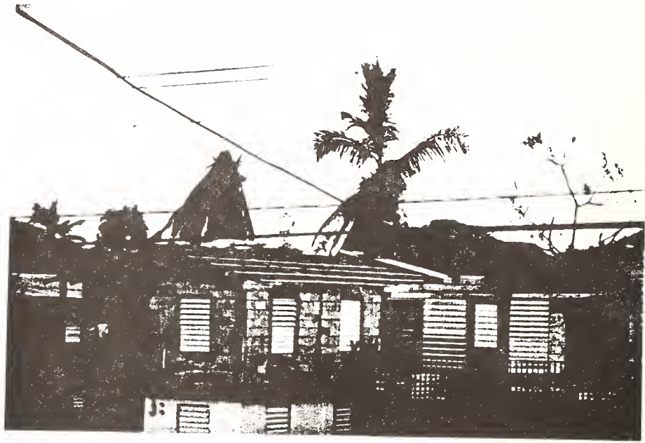
Figure 12. Failed corrugated steel sheet roofing, Puerto Rico
