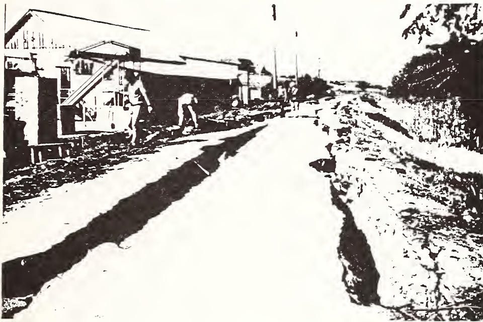
Figure 15. Liquefaction-induced fissures in levee of the Pajaro River, near Watsonville. The fissures were deeper than the height of the levee.
