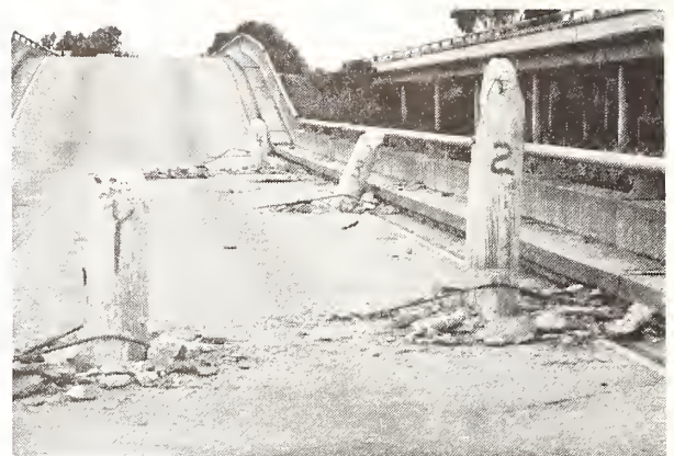
Photo. 10 4 Pile bents punched out (up to 1.2 to 1.8m) through slab at Struve Slough bridge.
