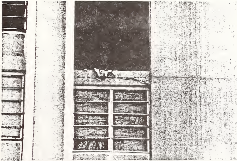
Figure 10. Damaged edge beams, concrete highrise buildings Fajardo, Puerto Rico
