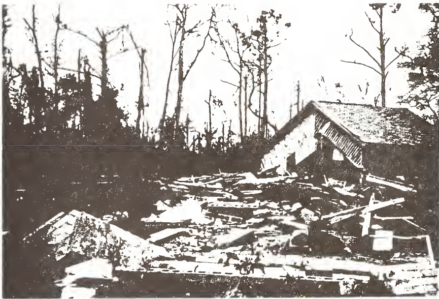
Figure 3. Shear Failure of House, Bull Bay.
