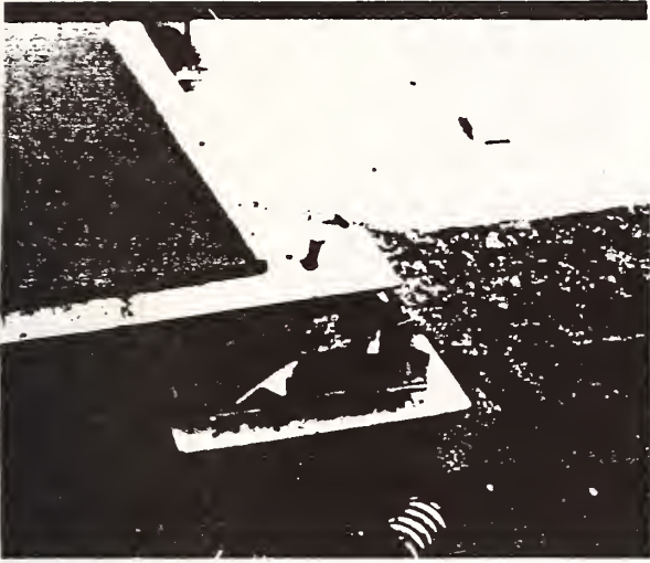
Fig. 1. Failure of Vibration Isolator, Watsonville Community Hospital
