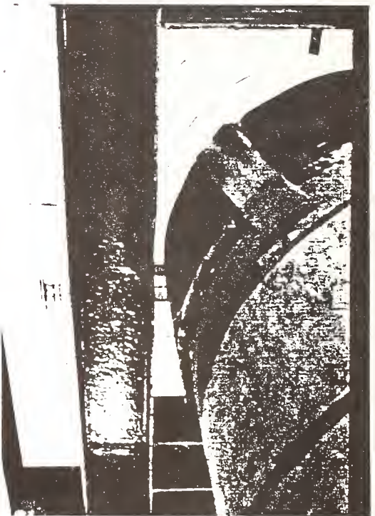
Fig. 8. Laterally Deformed Support at Moss Landing Power Plant
