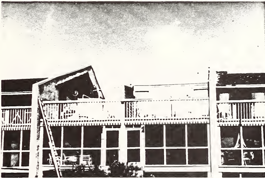
Figure 5. Condominium Roof Failure, Isle of Palms.
