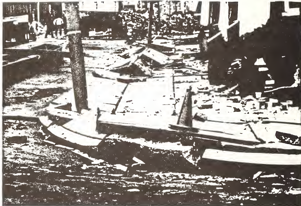
Figure 11. Buckled and broken sidewalks and street pavement resulting from soil liquefaction, in the Marina District.
