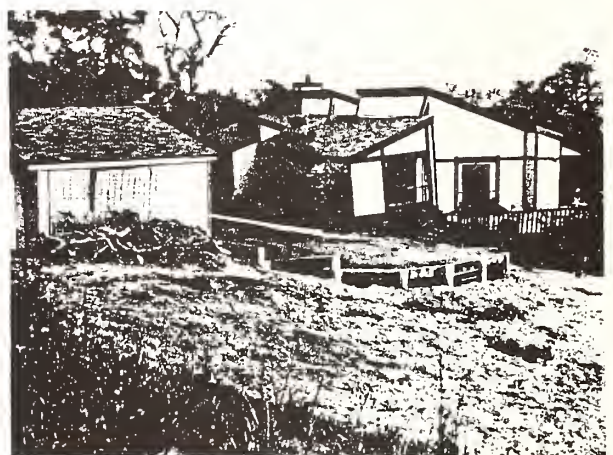
Figure 12. A badly damaged house in the Los Altos Hills area, supported on poles. The few connections between the poles and the floor framing failed due to poor quality welds. The floor joists were steel under the center portion of the house and wood at the edges. There appeared to be a lack of continuity between the two types of framing.
