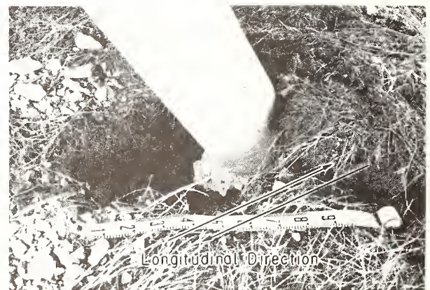
Photo. 12 Pile bent largely moved, causing a big hole surrounding the bent. Peat soils of high water content with high water table of 80 cm below the ground surface look very soft.
