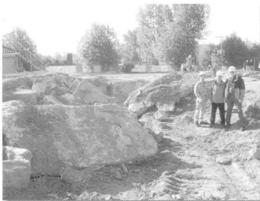
Family Housing Project Delivery Team members stand next to the old Japanese cement structure that was buried underneath the project site. This is one of the newest modifications to the project.
