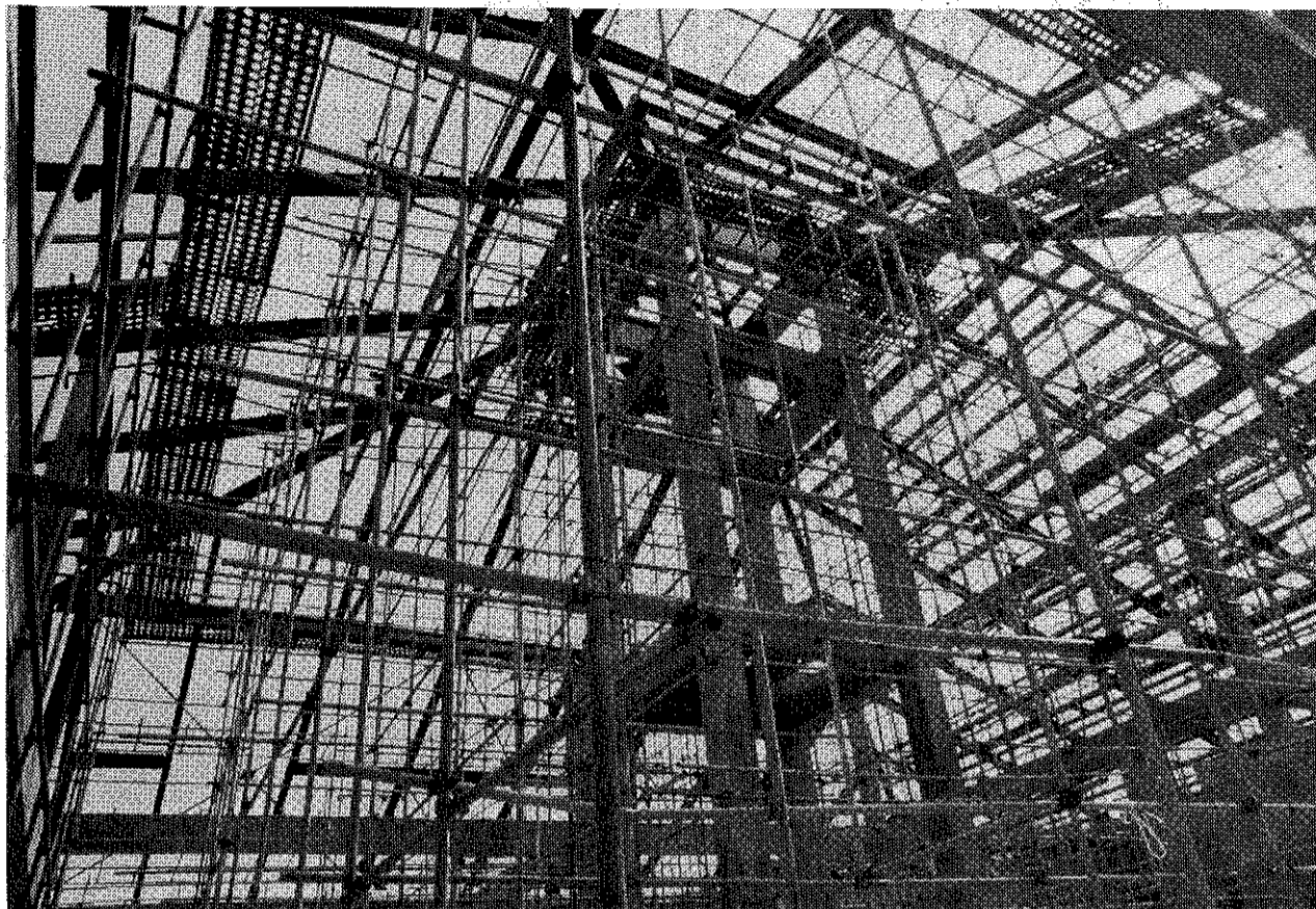
The roof construction for Yongsan Main Post Club requires careful safety. This project, constructed by Ssang Yong Construction Co., Ltd., is scheduled to be finished by next March.
