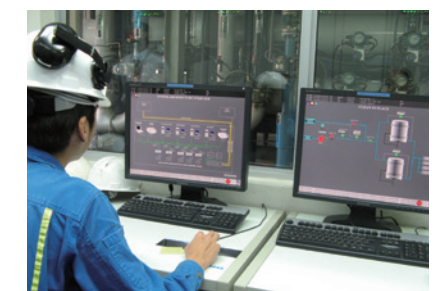
Main control room for field operations
