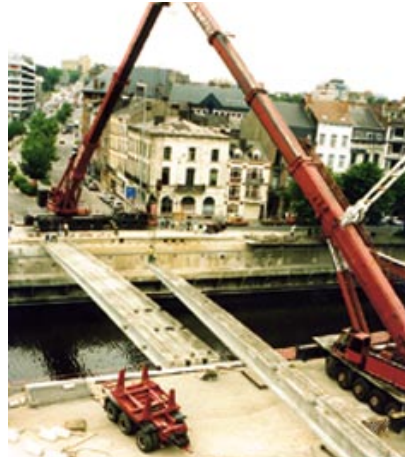
Infrastructure building, i.e. bridges, tunnels and railway sleepers, forms a considerable part of Partek's precast concrete production. In the picture, beams for the Pont de la Résistance bridge made by Partek's Belgian subsidiary are installed in the city of Charleroi in Belgium.
