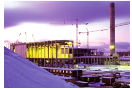
During 1994 and 1995 Partek Betonila delivered the concrete frames for the pulping line, drying section, bale storage facilities and wood room, and part of the wall elements for Metsä-Rauma's new pulp mill. This was the first time precast floor planks were used for casting the floors on which the machinery is installed, which speeded up the work and shortened the construction time.
