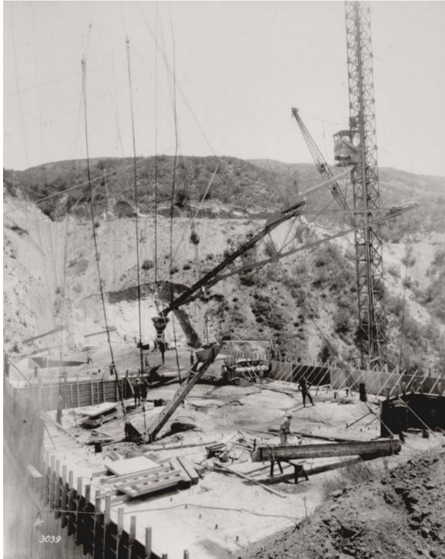
Figure 7. View looking west southwest towards the left abutment, in the Pelona Schist. Excavation of about 20 feet of schist can be seen, as well as the planar nature of the foliation surface, paralleling the abutment. Note the standing ponds of laitance moisture sitting upon the concrete pillows in foreground. Photo from L.A. Dept. of Water and Power.
