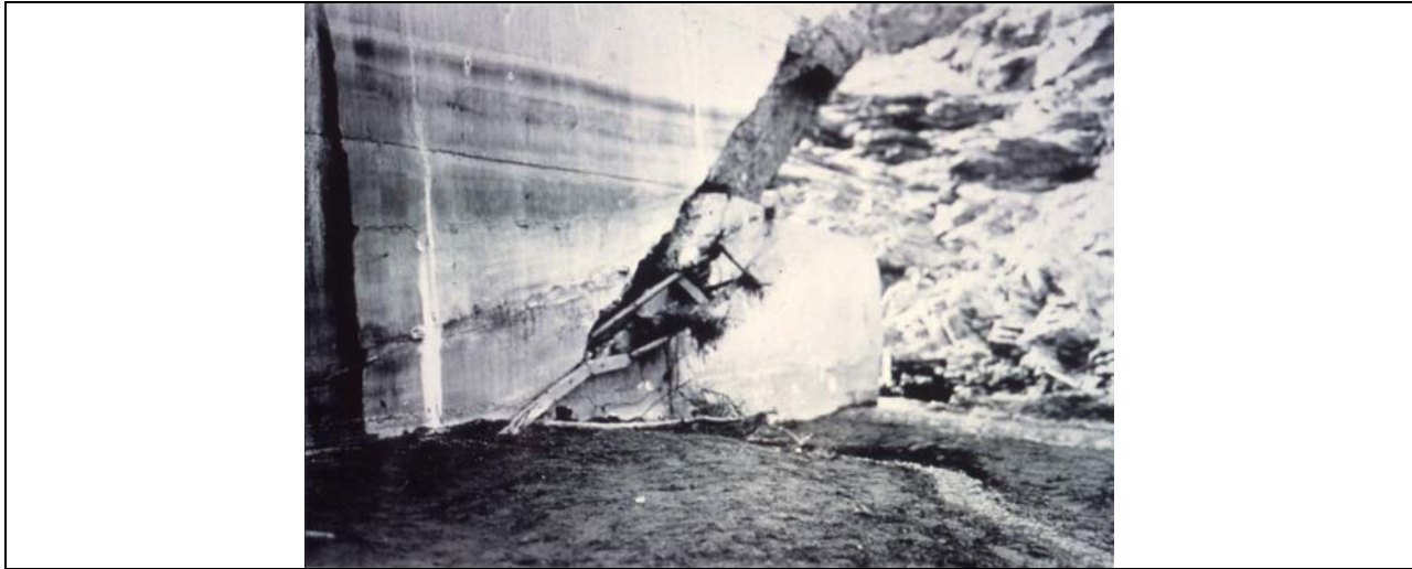
Figure 18. Detail view of the wooden gage attendant's ladder found in a large tension crack in the right upstream heel of Block 1. This testifies to significant deformation of Block 1, tilting downstream under active hydrostatic pressure. Some of this may have occurred after Block 2/3/4 fell away, removing lateral restraint on the left side of Block 1. Photo taken from Outland (1963).
