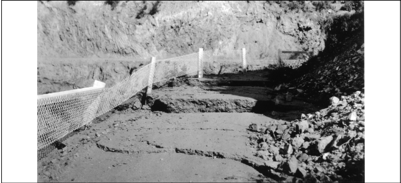
Fig. 11 - En-echelon tension cracks in San Francisquito Canyon Road several hundred feet upstream and about 20 feet above the dam's left abutment. The Ray Silvey family noted that one of these scarps was 12 inches high when they passed the dam between 8:30 and 9 PM, forcing them to stop their car and excavate ramps for their tires. These scarps were developed in the Pelona Schist. Photo by Bailey Willis, from the St. Francis Dam Disaster Collection at the Huntington Library.
