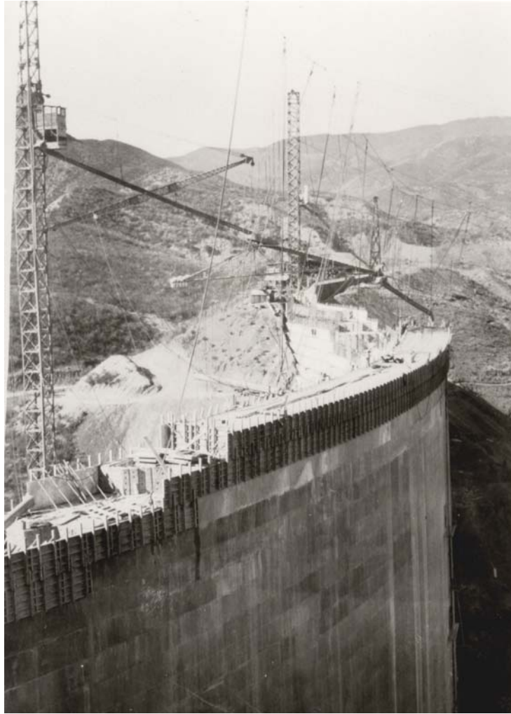
Figure 9. The dam design was amended to increase the overall height by 20 feet, taken in 10-foot increases on two occasions, a year apart. This view shows the dam topping out, sometime in 1926. The finished crest width was 16 feet. By this time the contractor was forced to install additional towers to aid in concrete placement along the dike section in the background. Photo from Lippincott Collection of U.C. Water Resources Center Archives.
