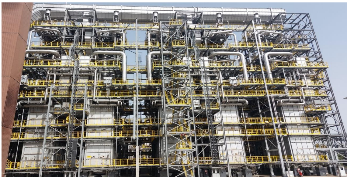
Figure 3. New pyrolysis heaters
