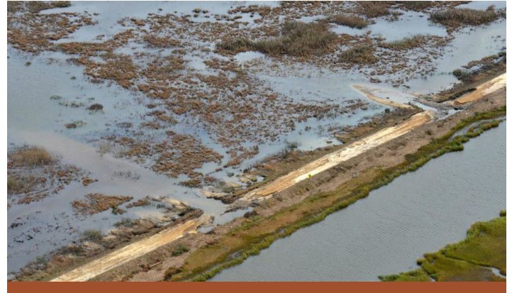
Storm-related damage to impoundments at Forsythe NWR in New Jersey. New Jersey Audubon Society
