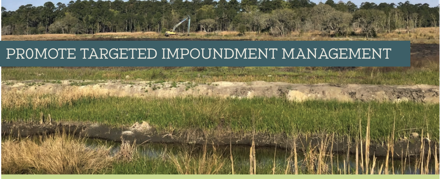
Cross dike construction for Black Rail management at Nemours Plantation, South Carolina. Nemours Wildlife Foundation
