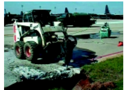
43rd CES personnel repair a 40-foot by 40-foot sink hole underneath the flightline taxiway, which was revealed the morning after Hurricane Floyd passed by Pope AFB. (Photo courtesy 43rd CES)
