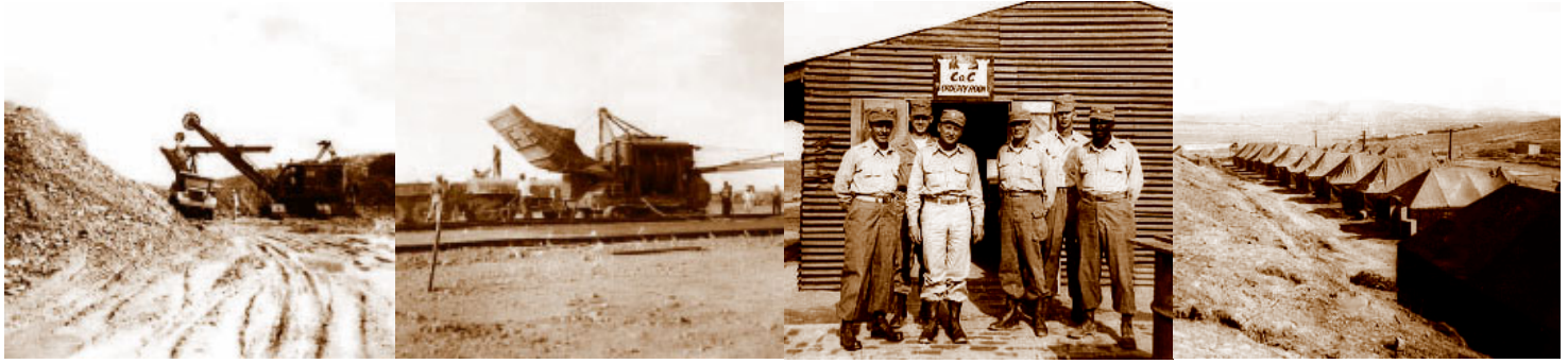
Snapshots provided by 1st Lt Fred Williamson (second from left in third picture) show the 839th EAB using power shovels to load gravel and rock into dump trucks for transporting to the rock crusher; loading crushed rock into a concrete mixer; officers of C Company, 839th EAB, in front of the company orderly room; and one of the rudimentary Army camps where aviation engineers lived. Camps were composed of squad-sized tents for enlisted personnel and metal buildings for company orderly rooms, battalion and group headquarters, officer quarters, mess halls and armories.
