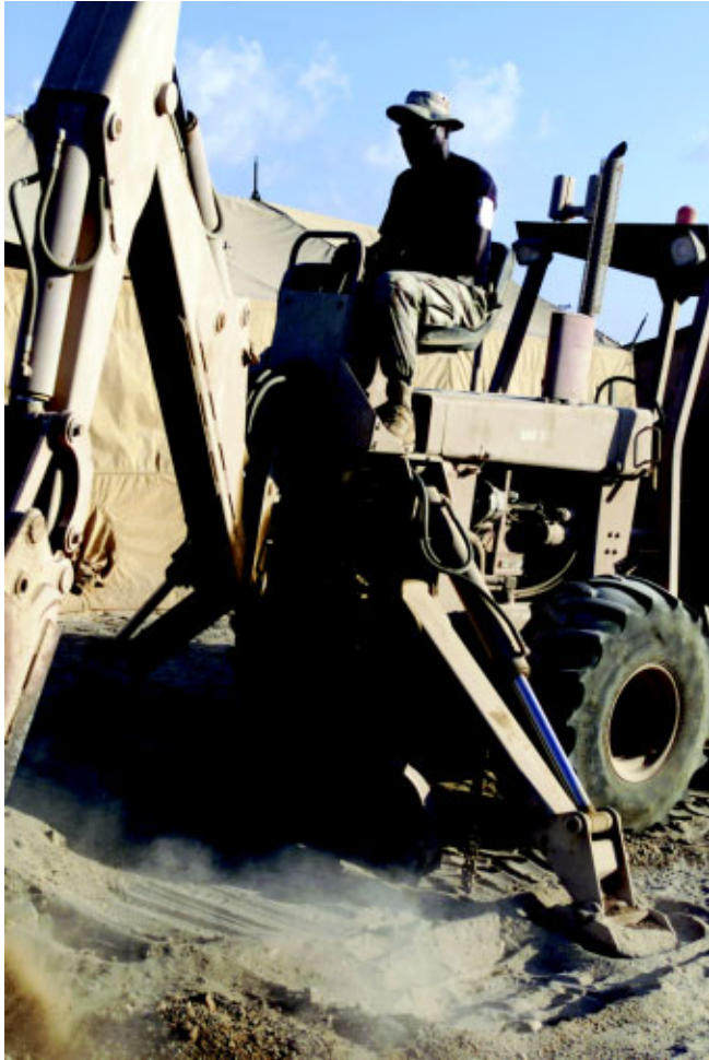
A CE staff sergeant excavates a trench so that drainage pipe can be laid at an undisclosed forward operating site Nov. 18. (Photo by MSgt Thomas Cook)
