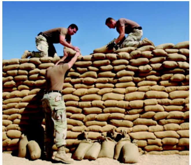
405th Air Expeditionary Wing firefighters add sand bags to a security wall at a deployed location Jan. 5. (Photo by SSgt Shane Cuomo)
