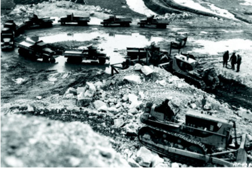
(Above) 1903rd EAB engineers haul rock from surrounding hills to be crushed for use in airfield and road construction. The greatest single day haul for the 1903rd as of March 1952 was 855 truckloads.
