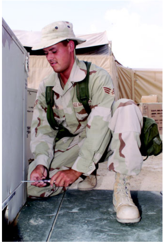
SrA Robert Keatts opens an environmental control unit for repair on Nov. 15. Airman Keatts is a deployed member of the 366th CES. (Photo by TSgt Michael R. Nixon)
