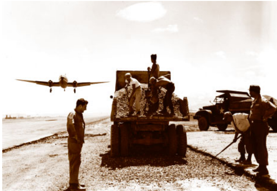
Members of the 811th EAB barely take notice of a C-46 Commando coming in for a landing as they work on a runway overrun.
