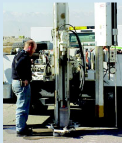
TSgt Steven Russell uses the automated dynamic cone penetrometer for pavement tests in Kabul, Afghanistan. (Above, right) The team goes to work at Kandahar International Airport. Members dressed to blend in with local Afghans.
