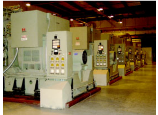
A total of seven diesel generators make up Schriever’s power plant and produce an astounding 16.5 megawatts of power.
