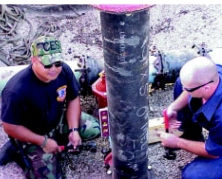
(From top to bottom) The pit of well number 1 on Aug 4, 2001. This is where Randolph's water contamination problems began. (Photo by A.C. Thomas) SrA Shaun Ballor, 37th CES equipment operator, stands by as emergency repairs are made to Randolph's water lines. (Photo by CMSgt Kenneth Thomas) TSgt Duane Cruz (left), 12th CES, and TSgt David Riggs, 37th CES, repair a section of broken pipe. (Photo by CMSgt Ercilia Ramos)
