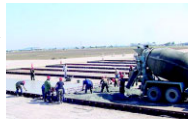
Craftsmen pour alternating concrete pad sections for Kunsan's hazardous cargo marshalling pad. The 554th completed the $475,000 project in 2001.
