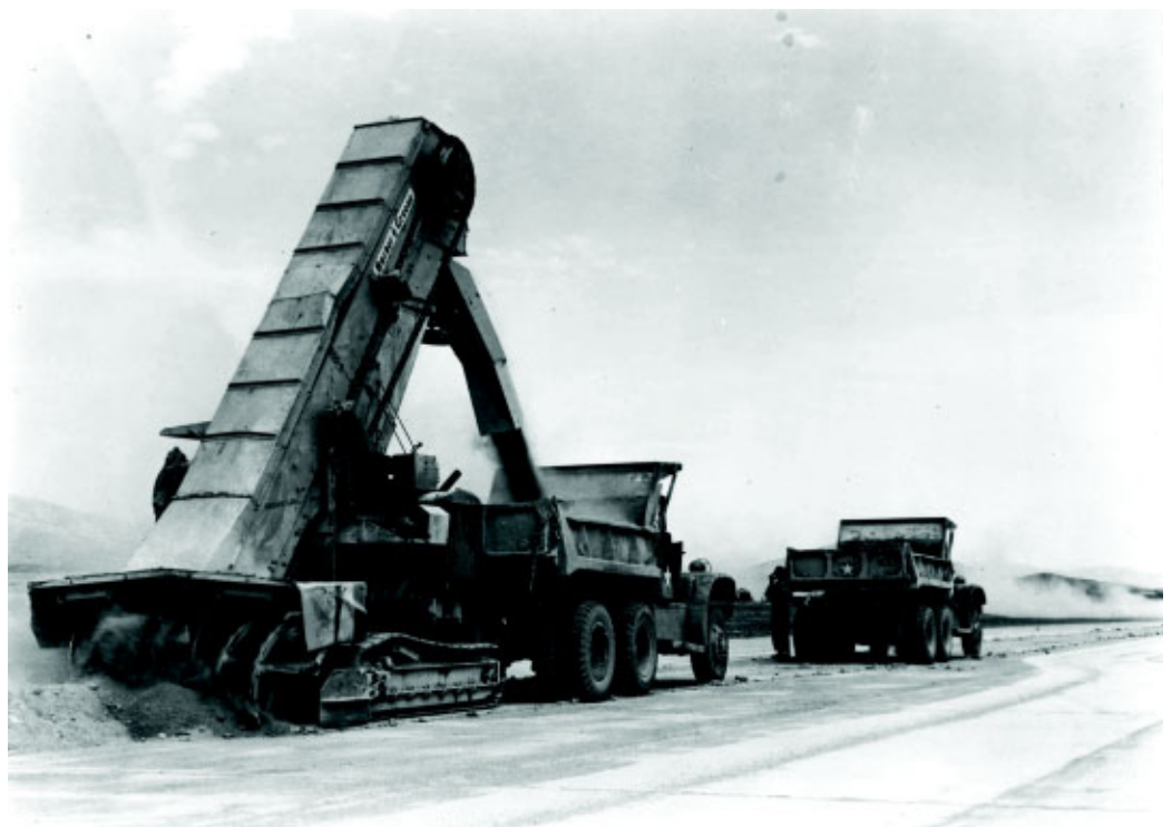
Trucks use a self-propelled conveyor loader to remove the curing sand from a 9,000-foot runway completed by the 930th EAG.
