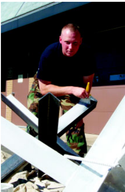
SSgt Alan Vanguilder, 148th CES, Minnesota Air National Guard, paints one of several newly constructed “road jacks” Oct.1. The Wing’s CEs constructed numerous jacks for use on roadways to provide enhanced protection for the resources and personnel supporting Operation NOBLE EAGLE. (Photo by MSgt Dean V. Kuhlman)
