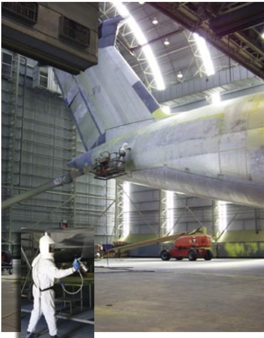
An end cap was added to this large-aircraft paint barn to accommodate the C-5's tail. "Cherry pickers" raise workers up to prep and coat the surfaces. In the new facility at Robins AFB, permanent manlifts will accomplish that task. The inset photo shows a closer view of the PPE described in the "Staying Safe" sidebar. (U.S. Air Force photos)
