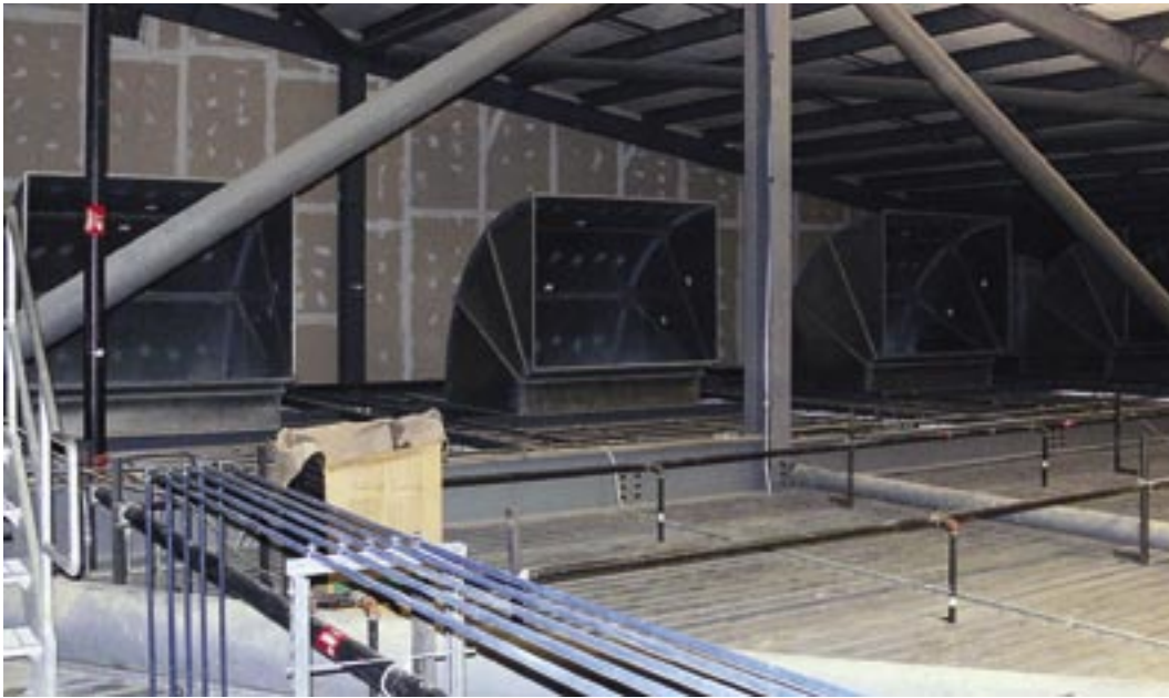
The interior of the overwing structural space is designed as a “duct.” Air from the recirculation fans — delivered through ducts visible at the rear of the photo — flows the length of the hangar before descending into a plenum (where it is mixed with conditioned intake air) and then into the hangar. (photo by Mr. Richard Kavanaugh, U.S. Army Corps of Engineers)
