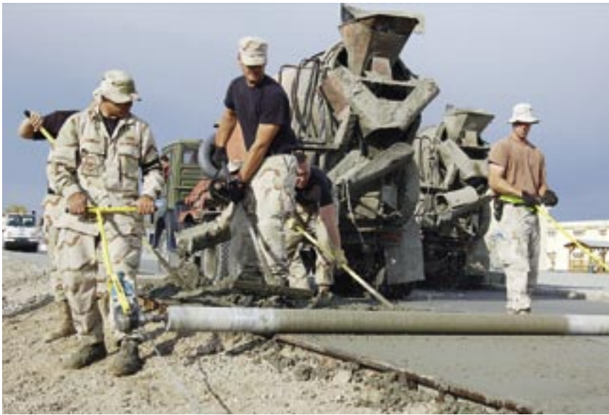
Members of the 376th ECES “Dirt Boyz,” SSgt Jeffrey Trombley (left) and TSgt Bryce VanOverbeke screed freshly placed concrete on a sidewalk, while SSgt Adam Ruter (center) rakes the concrete level. SSgts Trombley and Ruter are deployed from Grand Forks AFB, N.D., and TSgt VanOverbeke is deployed from Elmendorf AFB, Alaska. (photo by the author)
