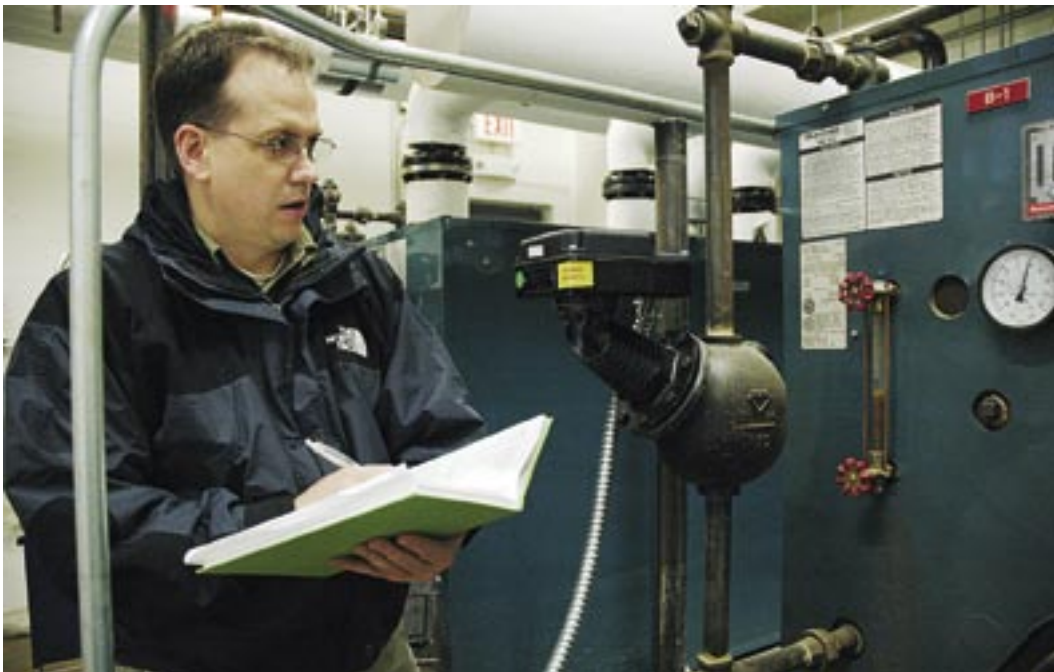
Mr. Eric Penland monitors boiler pressure at Elmendorf AFB, Alaska. (photo by Mr. Michael Forcht)
