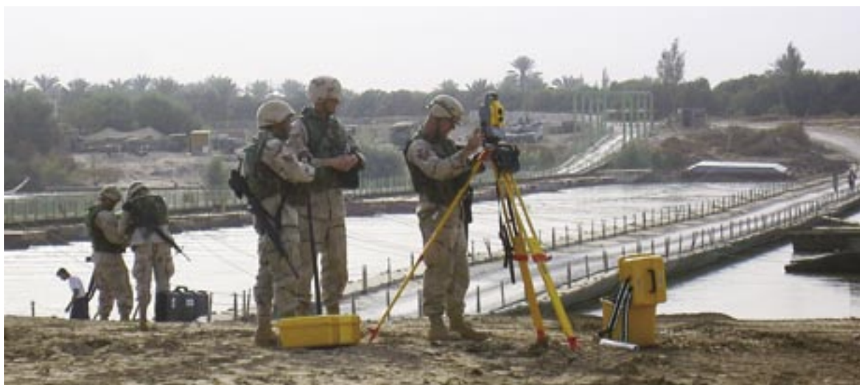
Members of the 240th CEF joined Active Duty engineering assistants to help the U.S. Army build bridges in Iraq. These two float bridges give civilians and coalition forces an important river crossing. (photo by Maj Phil Landeros)
