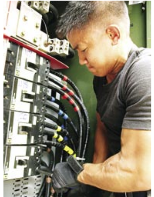
A1C Alex Jaime wrestles an electrical cable into place in a de-energized transformer on Wake Island. He's part of the damage assessment team sent to inspect the island following Super Typhoon Ioke. (photo by the author)
