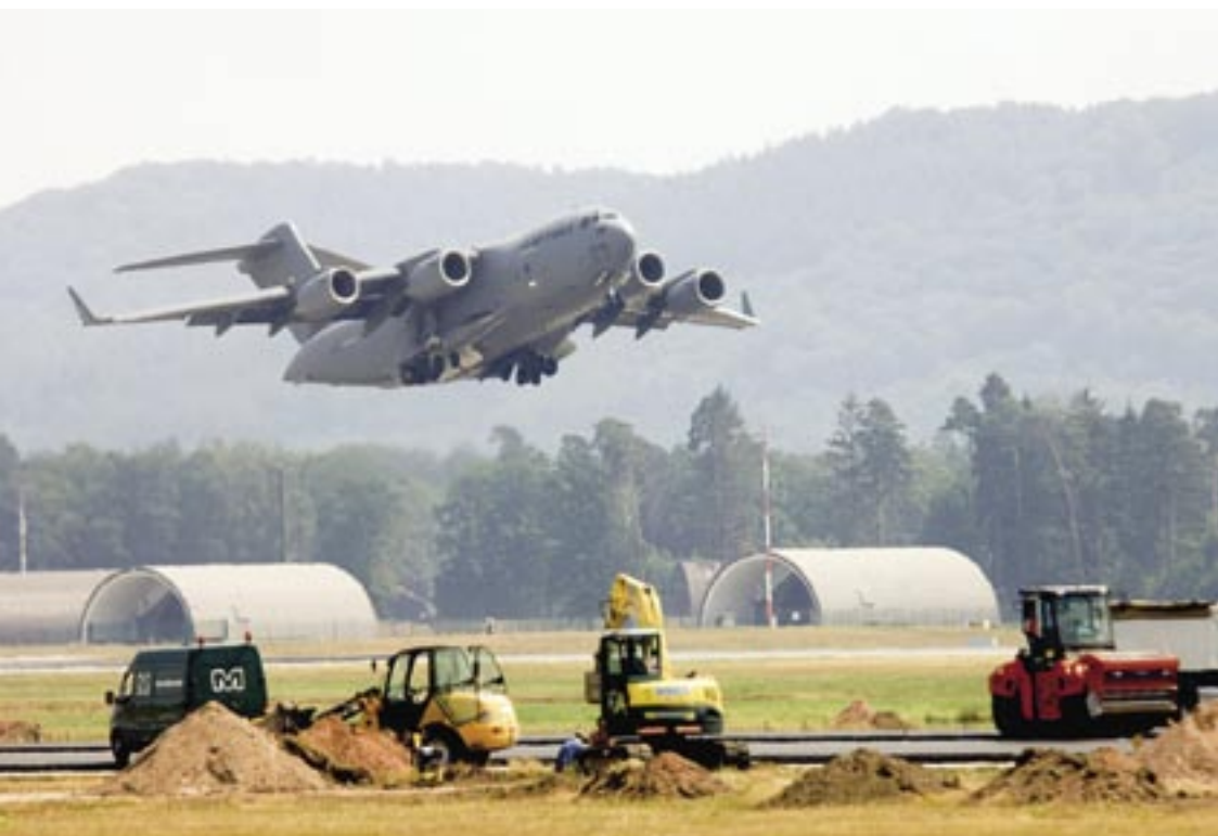
A C-17 cargo aircraft takes off from the south runway at Ramstein AB as construction continues to lengthen the north runway. (photo by the author)
