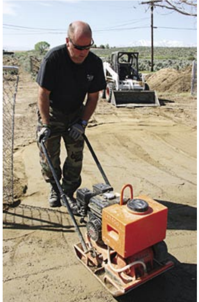
TSgt Cory Gillas, 939th CES, Portland, Ore., compacts the ground before building the frames and pouring concrete to make sidewalks at the Washoe Indian Reservation’s Head Start building. (photo by the author)
