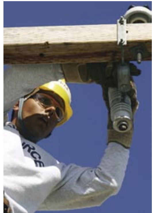
A competitor works to replace an insulator during the Lineman's Rodeo. (story and photo by SrA Tonnette Thompson, 82nd TRW/PA)
