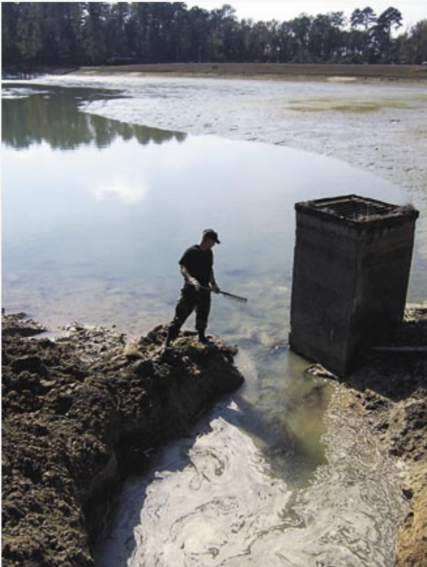
Left: TSgt Robert Wyatt, 78th CES, Robins AFB, Ga., clears obstructions from a drain pipe at Luna Lake. The 8.25 acre lake was drained of 12 million gallons of water to allow installation of a new siphon overflow system. Photographer: Ms. Redith Lee. Camera: Kodak DX-7440.
