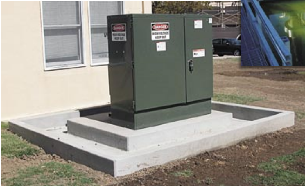
Containment curbs can impede electrical workers' access to—and egress from—transformers. They can also fill up with rainwater, which becomes stagnant and unsanitary, adding a recurring manpower burden for monitoring, sampling, and draining. (U.S. Air Force photos)
