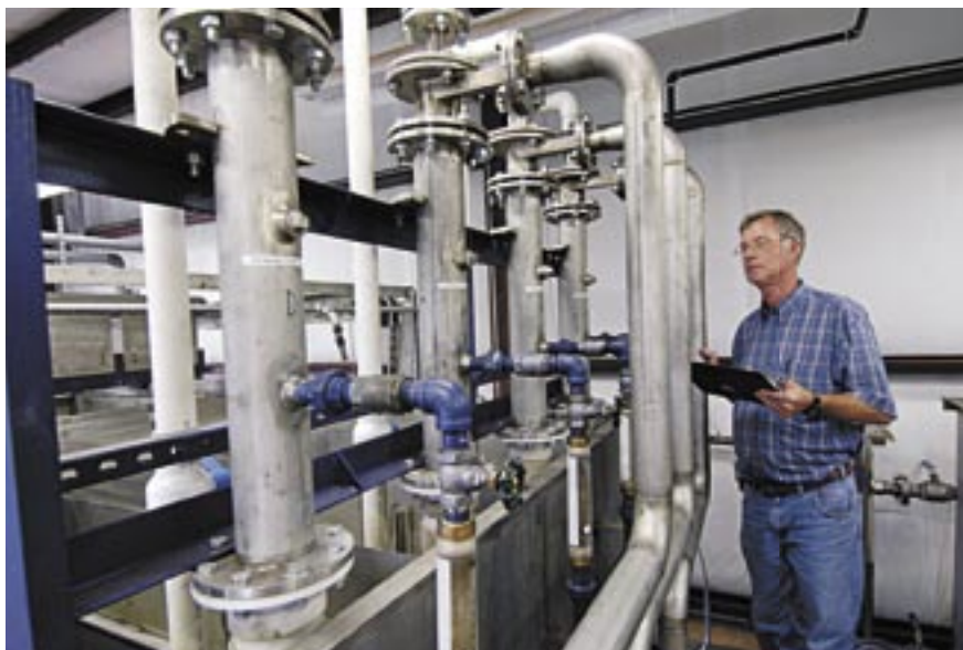
Mr. Bill Clark looks over new vertical hydrocyclone tubes, the beginnings of four stages where forced air aids in cleaning Tinker's industrial waste water at a rate of 144,000 gallons a day. (Photo by Ms. Margo Wright)
