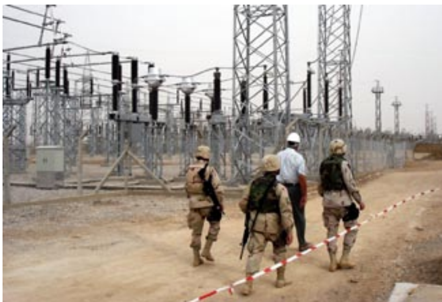
North Central Iraq RROC members tour a power generation facility in Kirkuk after the installation of a new 65mW generator. (U.S. Air Force photo)
