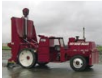
Left: The guillotine breaker cracked the pavement into 12"-15" pieces. Center: The multiple-hammer breaker—with up to 16 separate, 1,000-1,500 lb. breaking hammers—broke the chunks from the guillotine breaker into 6" pieces. Right: The Z-Grid roller seated the rubblized concrete and vibrated the pieces into a stable base. (photos courtesy Applied Research Associates)
