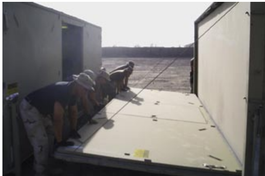
A team lowers the floor panel and vertical wall that supports the roof and ties the side walls. (photo by SrA Dora Sherrill)
