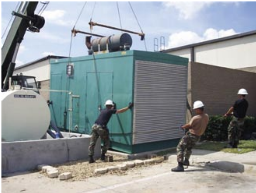
AFCEA's CEMIRT transported three 500 kW generators from Tyndall AFB, Fla., to Keesler AFB, Miss., immediately after Hurricane Katrina and installed them to provide much-needed emergency power. (photo by Mr. Timothy Collins)
