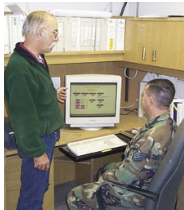
Chuck Moler, EMCS Manager, shows TSgt Craig Spicer, HVAC Craftsman, the EMCS station for hands-on control from the HVAC shop. Any shop standby member can verify the auto shutdown plus restart specific facilities or areas of base from this terminal. (U.S. Air Force photo)
