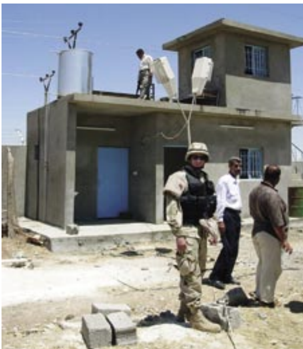
POInT member CMSgt Cevin Cox conducts a final inspection on a guard-house and tower facility at the Mullah Abdullah Power Plant. (photo by the author)
