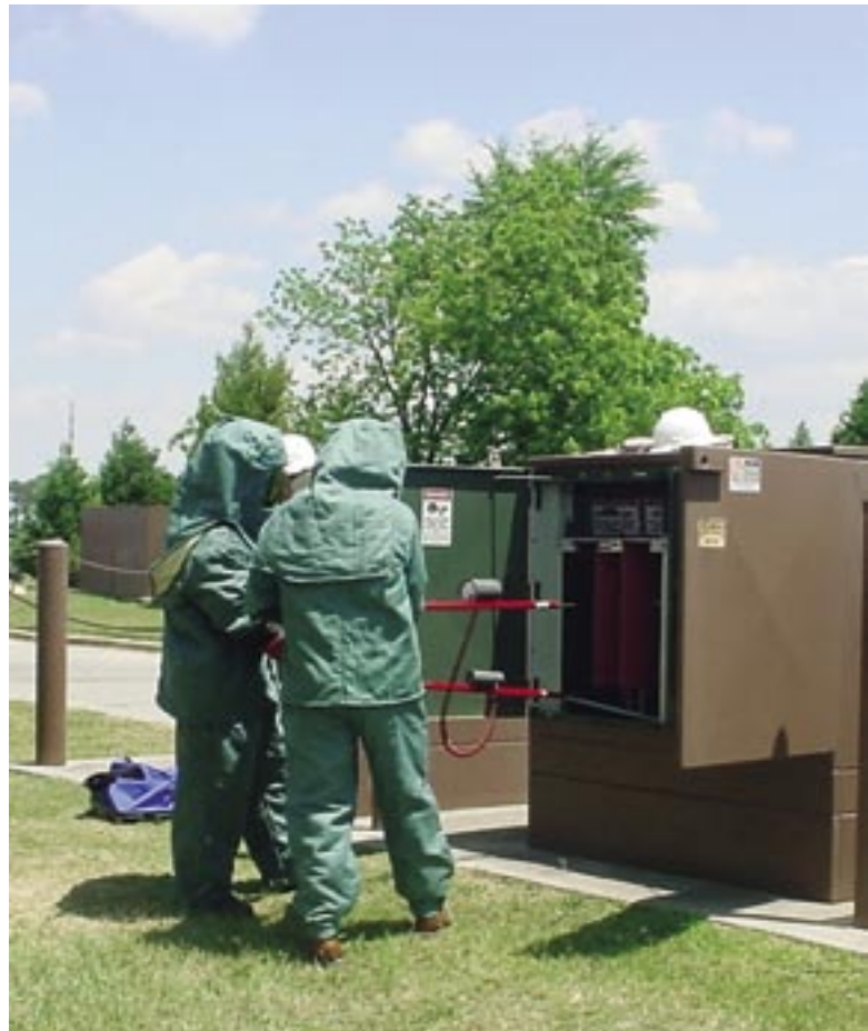
Mr. Bobby Rhodes and Mr. Billy Bandy, electricians with the 78th CES, use the appropriate PPE to work on high-voltage switchgear. (photo by Mr. William Fowler)
