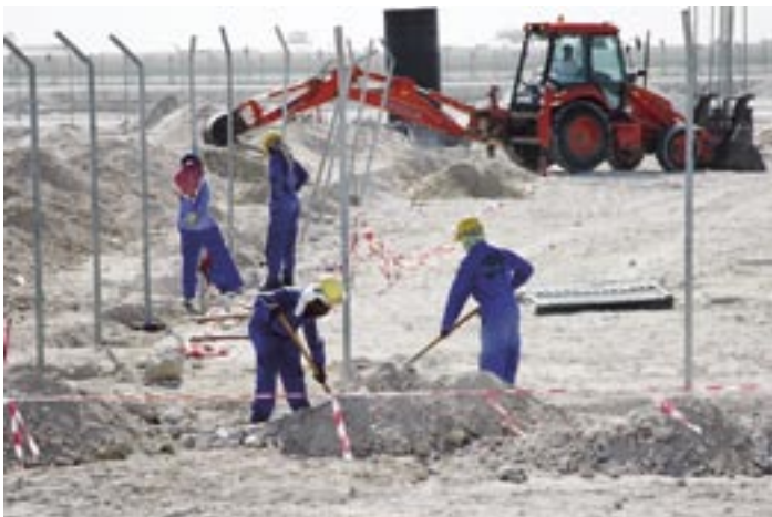
Contract workers build a perimeter fence for a new temporary cantonment area for the 380th Air Expeditionary Wing in Southwest Asia. (photo by Mr. Jerry Shumate)
