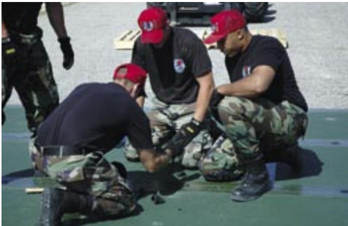
Although this fiberglass mat is very light, Det 1 of the 823rd RHS discovered that the locking pins don't fit unless the panels are perfectly aligned. (photo by Mr. Guy Ivie)
