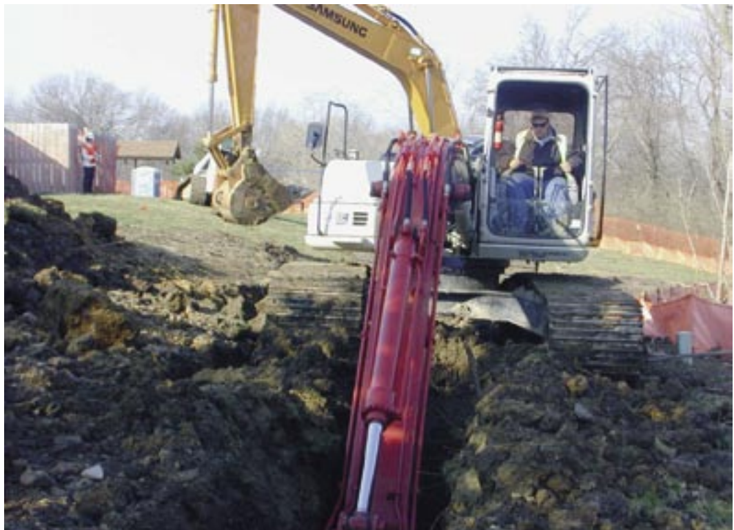
Trenches were dug to install the biowall at Whiteman AFB. (photo courtesy CH2M Hill)
