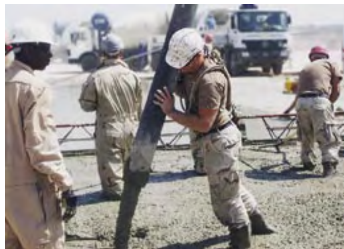
SrA Terrell Jackson (left) and SrA Andrew Hikes, 557th ERHS, direct a high-reach concrete pump during the heliport construction project in Southwest Asia. (U.S. Air Force photo)
