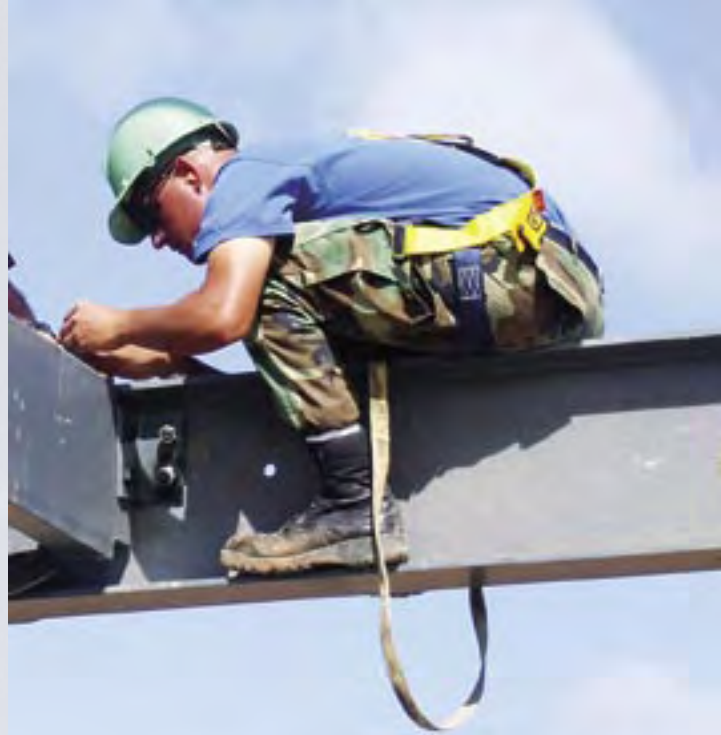
SSgt Johnson secures a mezzanine floor beam for the Police and Fire Emergency Substation. (photo by 1Lt Megan Poyant)
