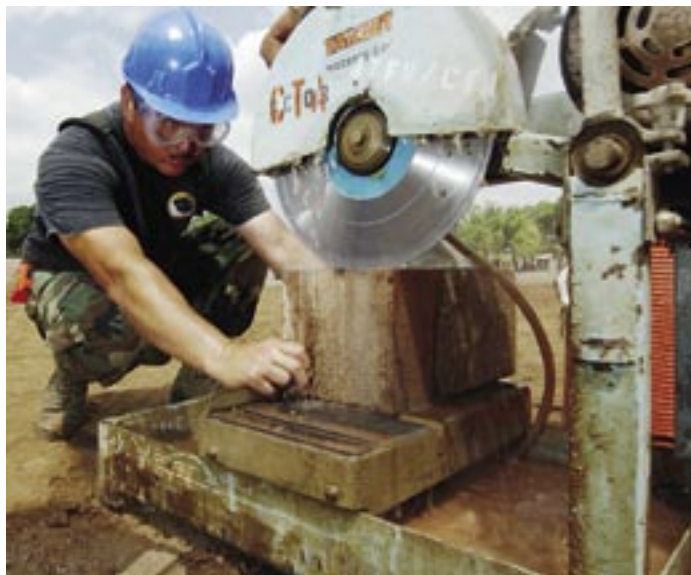
Top: SSgt Angela Kimble, 507th CES, Tinker AFB, Okla., and Capt Heidi Gaddey, 99th Medical Squadron, Nellis AFB, Nev., level concrete for a new school's foundation in Tecoluca, El Salvador. Center, left: SrA Brandon Tenney, 349th CES, Travis AFB, Calif., works on the flooring for lodging tents in La Mesa, Panama. Center, right: SrA Joshua Reyes, 349th CES, Travis AFB, Calif., surveys the base camp area in La Mesa, Panama. Bottom: TSgt Darren Kennedy, 507th CES, Tinker AFB, Okla., uses a masonry saw to cut bricks that an El Salvadoran Army soldier (right) will use for the walls of a new school in Tecoluca, El Salvador. (top & bottom photos by SSgt Reynaldo Ramon; center photos by Mr. Miguel A. Negron)
