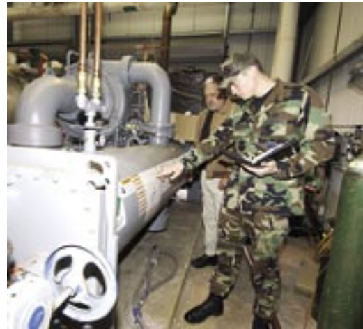
2Lt Desautels and Mr. Moore saved Tyndall AFB more than $160,000 by relocating this chiller. (photo by Ms. Lisa Norman)
