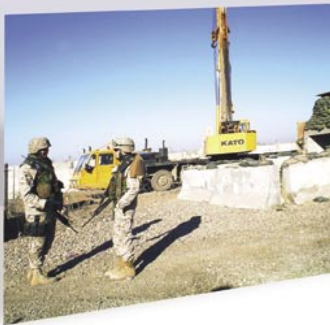
Above: All work outside the wire at Abu Ghraib Prison, such as moving these bunkers at the entry control point (ECP), is done under guard. Left: SrA Casey Feathers has gun duty as the vehicle enters the ECP. (photos by TSgt José Ortizfigueroa)
