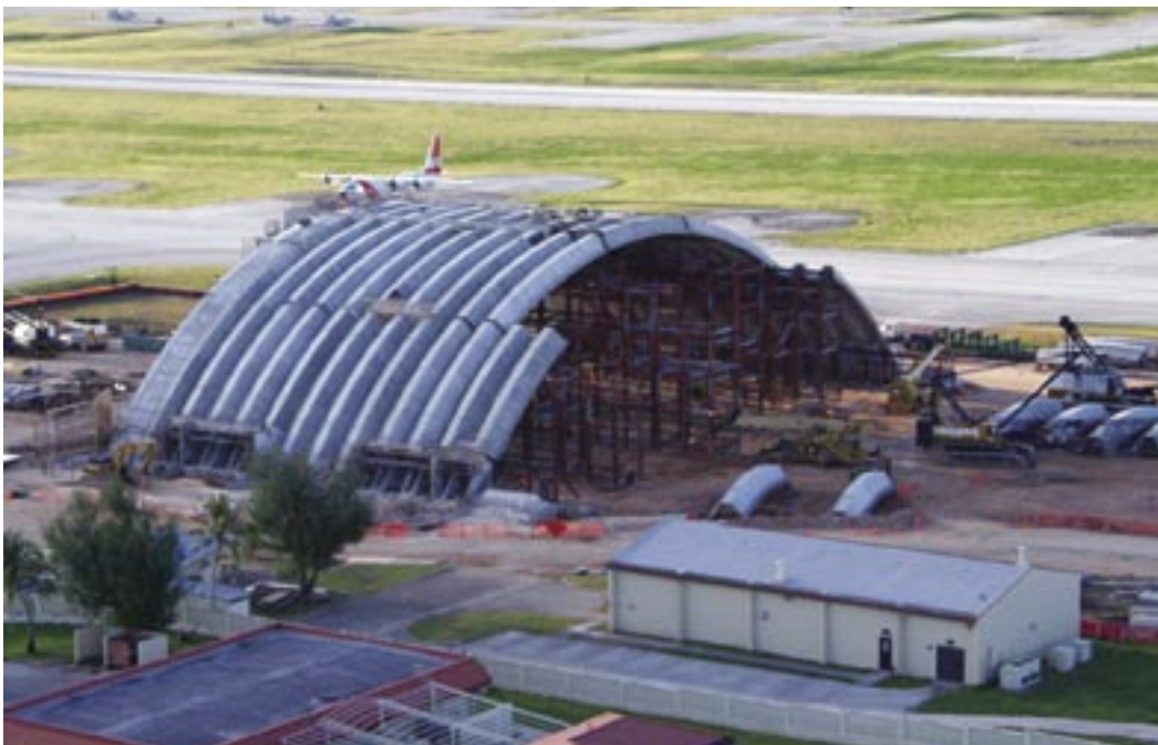
Work crews continue construction of the new forward operating location hangar at Andersen AFB, Guam. (photo by A1C Joshua P. Strang)
