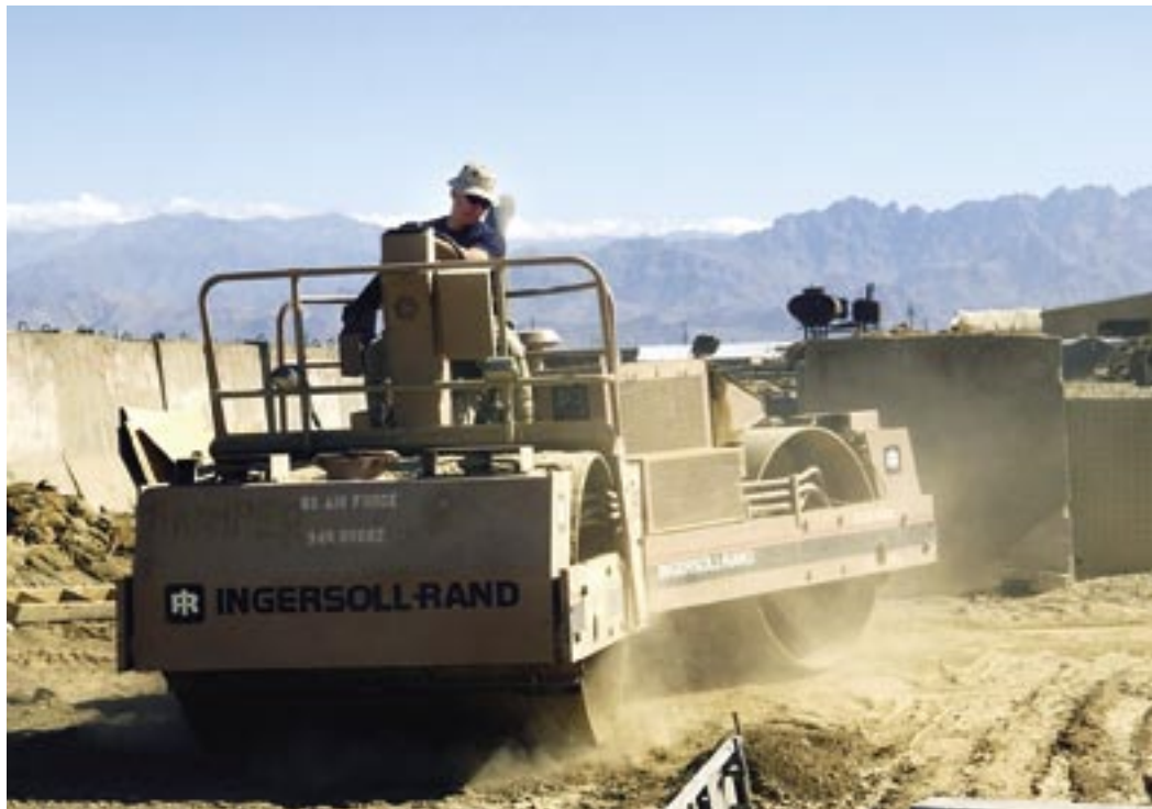
SSgt James Crosley uses a roller to pack down dirt before civil engineers pour a concrete foundation pad at Bagram AB, Afghanistan. Digging in the dirt here can be somewhat risky. In the past two months, the heavy-equipment team has found nearly a dozen old munitions, ranging from old fuses to rocket payloads and bombs. SSgt Crosley, on deployment from Kadena AB, Japan, is assigned to the 455th ESS. (photo by MSgt Andrew Gates)
