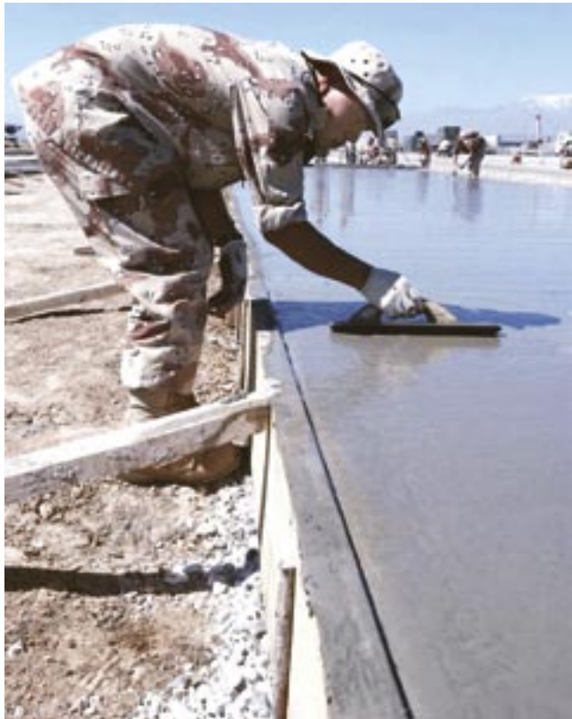
Pfc. Yi Dong Gon, an engineer with the 100th Korean Engineer Corps, puts the finishing touches on still-wet concrete on the Bagram flightline. (photo by the author)
