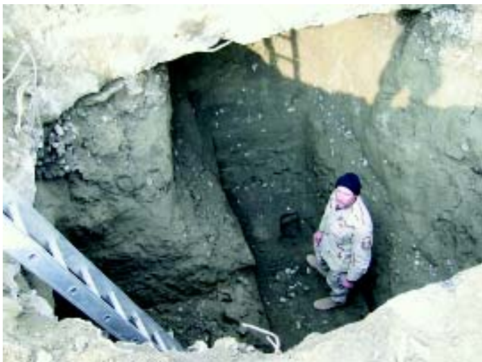
MSgt James E. Brewster, 379th ECES, stands at bottom of hole excavated to find the entry route of UXO located beneath runway in Afghanistan. (U.S. Air Force photo)
