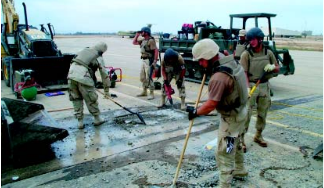
An ARH team repairs a spill on a runway at an Iraqi air base using equipment from the MARES: CAT 420 backhoe (left) and IHI IC-45 crawler carrier (right).
