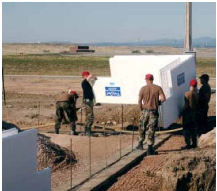
Above right: Windows were framed into this exterior wall. Below right: ICFs were sometimes formed off site and carried into position. (photos courtesy 819th RHS)
