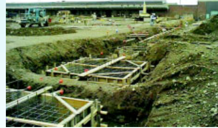
Construction crews begin work on the new, consolidated facility. The project will be completed in 2003.
