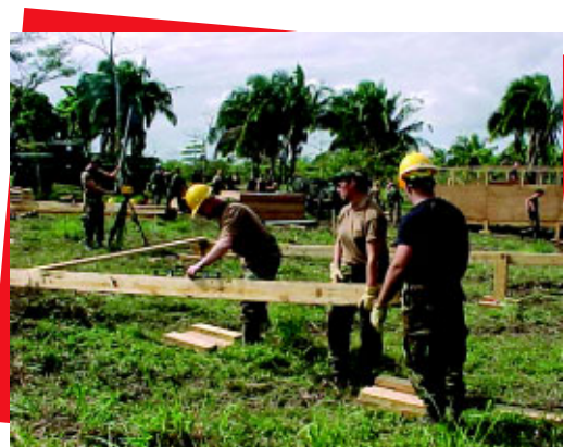
With work nearly complete on one hardback tent shelter in the background, teams begin setting up another. More than 22 such tent pads were constructed during the team’s two-week stay in addition to other infrastructure projects.
