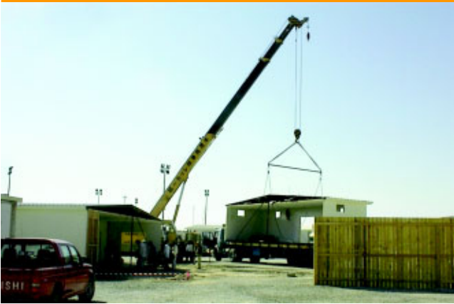
Civil engineers at Al Dhafra found that the most efficient way to erect buildings in that area of the world was to purchase modular ones and have them delivered to the site.
