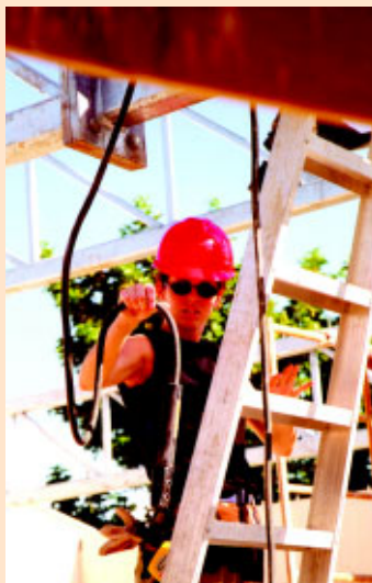
SrA Crystal Register works to put on the roof at the Jamaican Defense Force Barracks at Up Park Camp in Kingston, Jamaica. (Photo by SrA Stephen Hudson)
