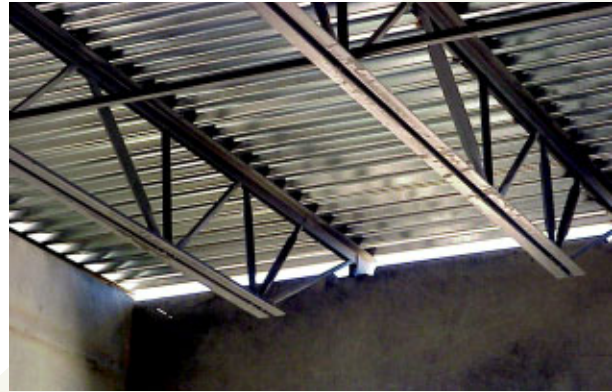
A crane was used to set the steel joists for the roof in place.
