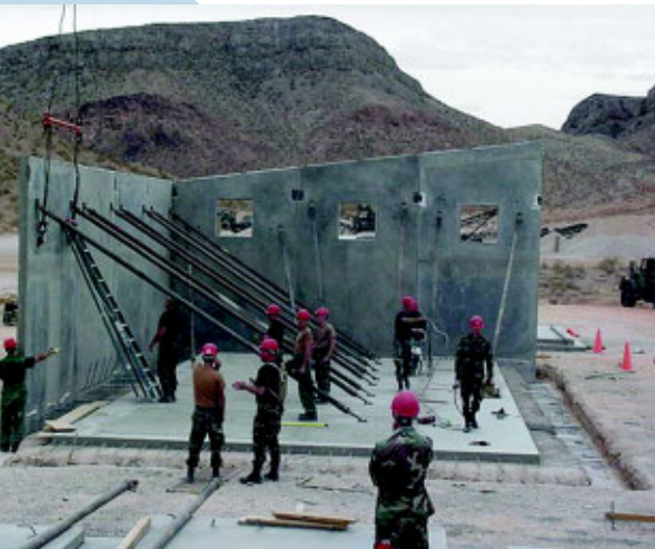
820th RHS members used the tilt-up method to construct a quarry maintenance facility on Nellis AFB. (Photos courtesy 820th RHS)
