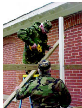
SMSgt Charles Anderson (on ladder), 153rd CES, and another member of the 153rd repair a fence on Warren AFB. (Photo by MSgt John Sandness)
