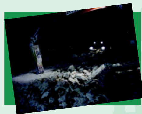
Photos show the 384th ECES team at work breaking rock in order to clear enough land to build a parking ramp to expand the flying mission at their forward deployed location. (Photos courtesy 384th ECES)
