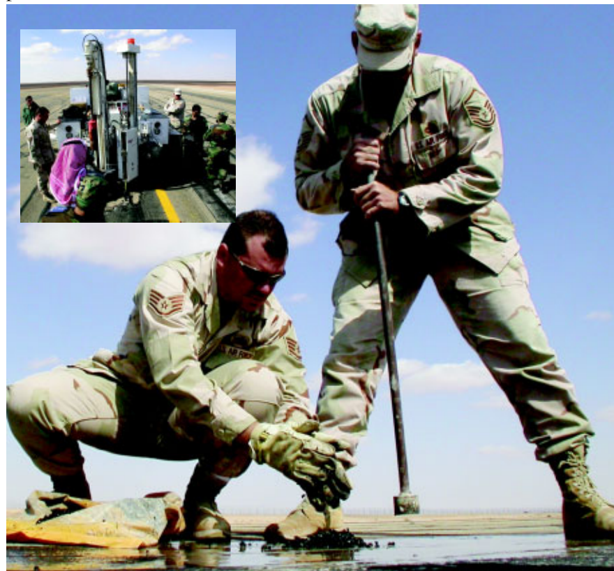
(Above and inset) MSgt Scott Melton and SSgt Greg Welch patch a core hole on an airfield as interested locals observe. Everywhere the team went, the local populace was curious about their work.
