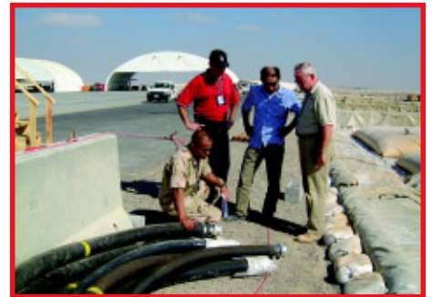
(Top to bottom) The 380th ECES broke ground Christmas Day 2002, excavating and grading land for a new fuel farm at their forward deployed location. Local contractors perform quality control checks on the piping system. Capt Juan Alvarez, 380th ECES Engineering Flight chief, and construction manager Ken Lombard of RMS worked with contractors to complete the project, which resulted in a wartime throughput averaging over 2 million gallons of jet fuel per day. (Photos courtesy 380th ECES)
