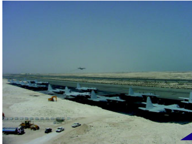
The SWA Delivery Team resolves planning, programming and construction issues for civil engineers in forward operating locations to expedite projects such as this aircraft parking ramp built by a Prime BEEF team for Operation IRAQI FREEDOM, and beddowns such as the tent city at Manas, Kyrgyzstan, below. (Tent city photo by CMSgt Andrew Stanley)
