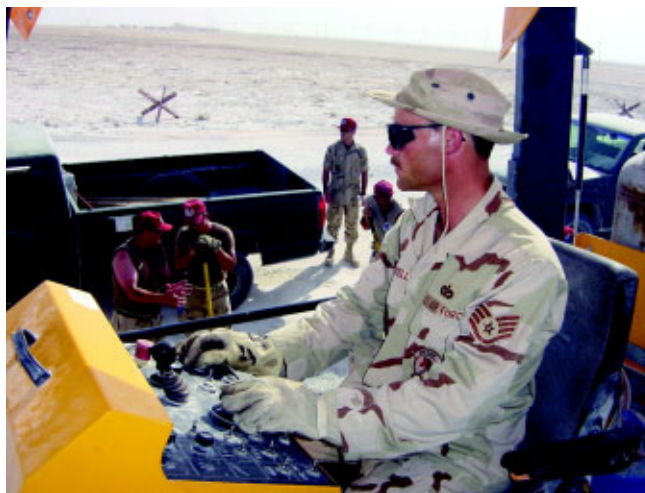
SSgt Chris Blackwell, a heavy equipment operator with the 200th/201st ERHS, operates an asphalt paving machine at Al Udeid AB. (Photo by A1C Tarkan Dospil)
