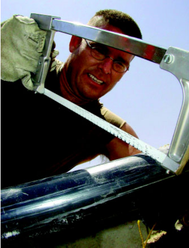
SSgt Todd W. Puckett, 200th/201st ERHS airfields section, cuts conduit for airfield taxiway lighting at a forward-deployed location. (Photo by A1C Joe Pearce)
