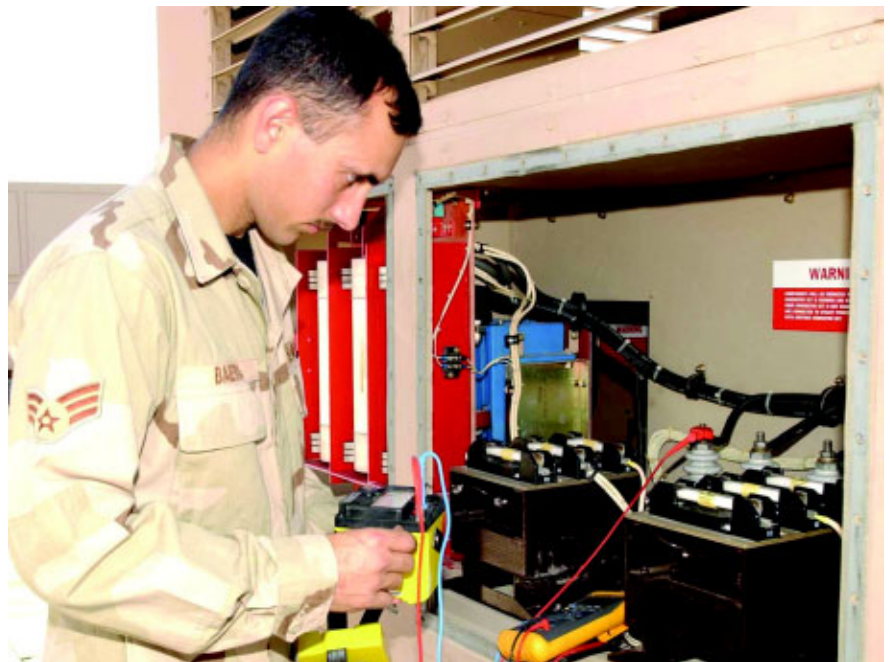
SrA Marco Baeira, 320th ECES, uses a megohmmeter to check for breakdown within a high-voltage step-down transformer (Photos by SSGT Pamela Smith)
