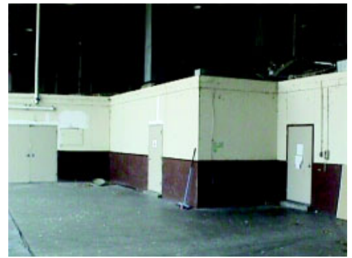
Hangar 5's floor was converted to office space for helicopter mission personnel in 1975 by anchoring modular sections within its bay.
