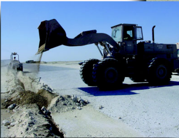
(Above) A1C Brady Dryden, 27th CES, dumps sand around a new water line that will tie the water plant to the dining hall at his deployed location.
