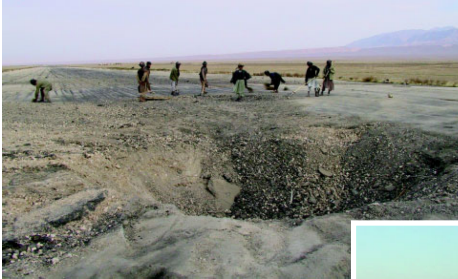
Afghan workers clear debris near a massive crater on the runway at Mazar-e-Sharif. Under the supervision of RED HORSE, the workers patched eight large craters on the runway.
