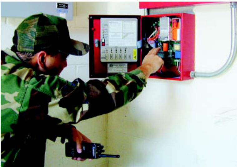
Nearly all civil engineer radio-based systems, such as the Monaco Enterprises BT2-3 fire alarm transceiver radio unit being examined by A1C Lance Carson, 325th CES, Tyndall AFB, FL, above, will be impacted by the NTIA narrowband mandate. (Photos by Dave Mathews)
