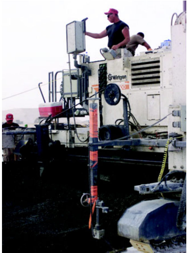
SSgt Chuck Risinger, 823rd RHS, operates a slip form paver March 24. SSgt Wayne Skocelas makes sure the surface of the concrete has enough moisture to obtain the proper finish. On the ground, MSgt Bizzle Davis keeps steering sensors clear from debris. (Photos by SrA Danielle Upton)
