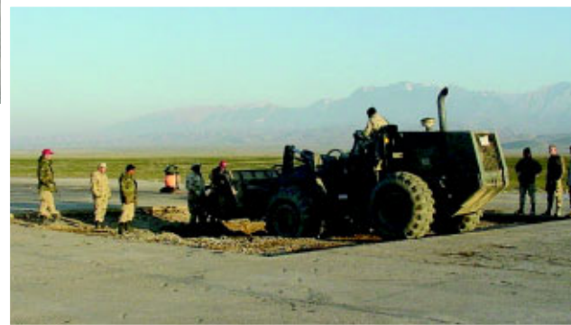
The team was able to get a deployable pavement repair system on site in January. Pictured is SrA Cleofies White using a front-end loader to backfill the excavated crater.
