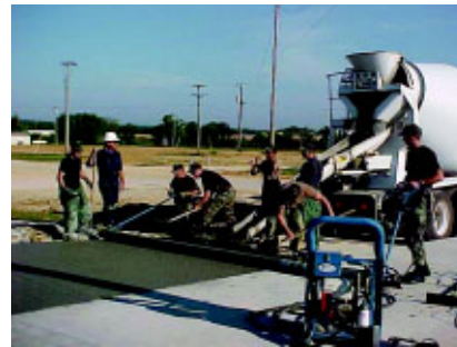
Pavement and Construction Equipment Operator instructors use a power screed to place and finish concrete for a self-help parking lot driveway at Ft. Leonard Wood. (Photos courtesy 366 TRS, Det 7)
