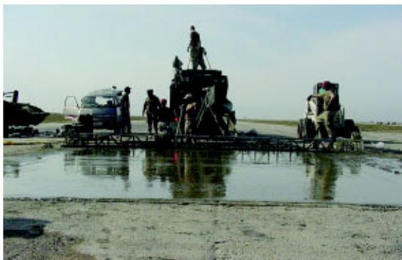
The team completes the second and final pour on one of the craters and finishes the concrete. At center, above, is the Deployable Pavement Repair System (DPRS) with members refilling the material bins.
