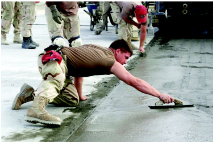
SrA Justin Soule, 823rd RHS, finishes the edge of a new 1,240-foot long concrete lane March 24 at Al Udeid.
