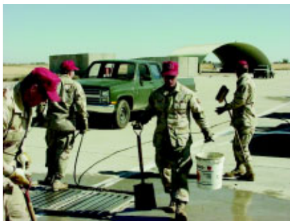
The 15-member team constructed a K-Span facility and repaired concrete airfield taxiways on the Israeli Air Force base.
