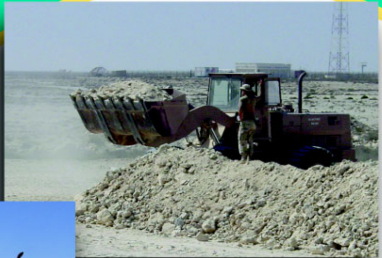
(Above) SSgt Dennis Rellins and SSgt Linwood Stull, both from the 27th CES, construct a holding facility for fuel. (Photos by Lt Col Nick Desport)
