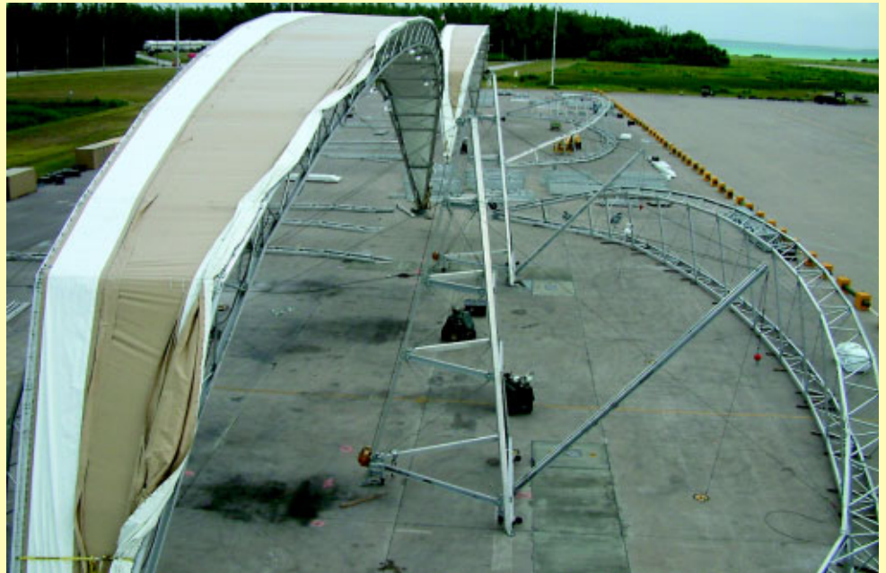
Dual construction towers (visible in front of first truss) were used to erect the B2SS. Both hangars were erected simultaneously.
