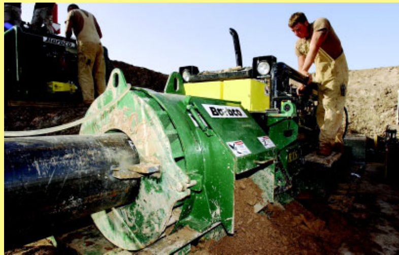
A1C Nathan Laidlaw operates a horizontal boring machine. The machine bores large holes for utility crossings under the airfield surface, eliminating trenching. (Photo by SSgt Tony R. Tolley)
