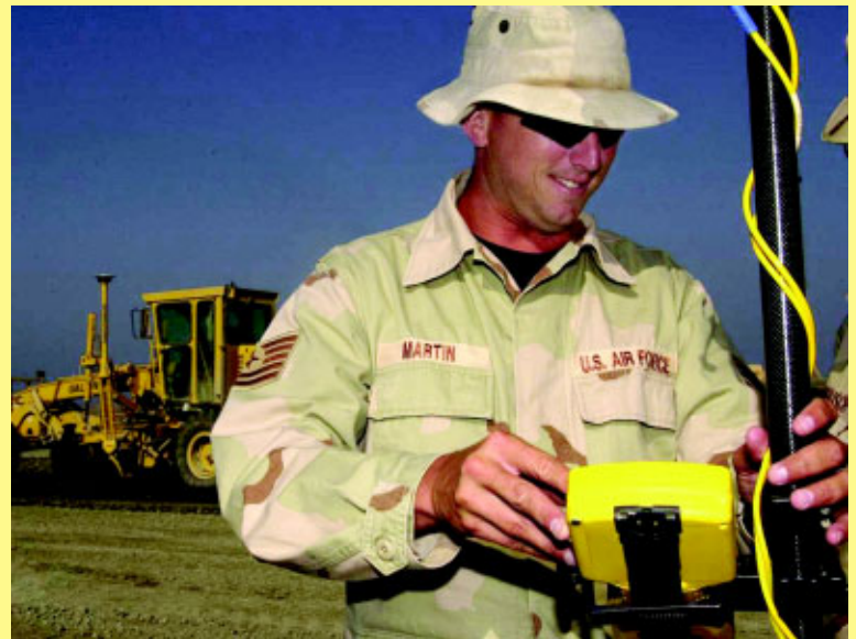
TSgt John Martin uses GPS to survey. Points are transferred to the GPS-integrated grader for construction. (DOD photo)
