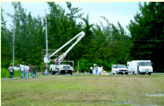
The local base operating support contractor at the deployed location helped CEMIRT make the final connection into the host nation power supply
