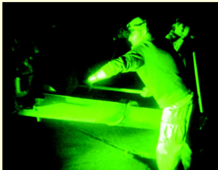
SSgt Scott McHugh, a heavy equipment operator, shovels concrete out of a chute during nighttime taxiway slab repair. (Photo by SSgt Bobby Yettman)
