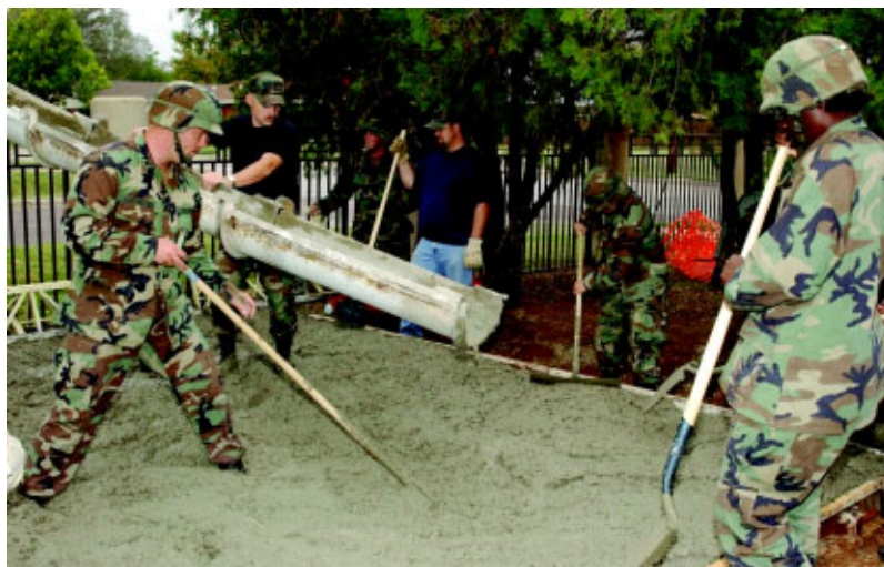
Members of both the 97th CES and the U.S. Army's B Co, 62nd Engineering Battalion pour a concrete pad for a storage shelter at the Altus Child Development Center. (Photos by Amn Richard Rose)
