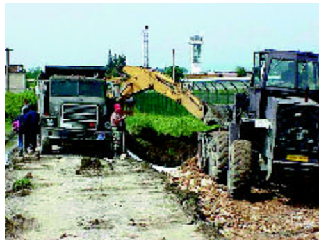
Perimeter road work at Rinas Airport, Tirana, Albania. (Photos courtesy 823rd RHS)
