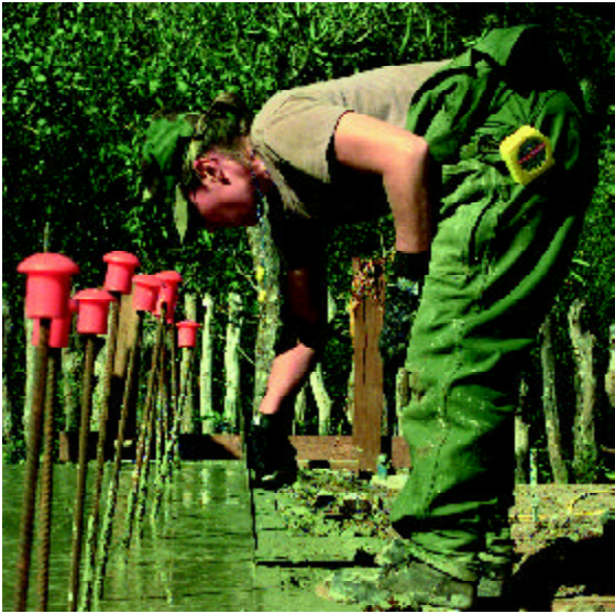
(Above) SSgt Amy Pope, 819th RHS, adds finishing touches to a concrete floor during construction of a two-room school in Camatindi, Bolivia. (Photo by TSgt Katherin Bryson)
