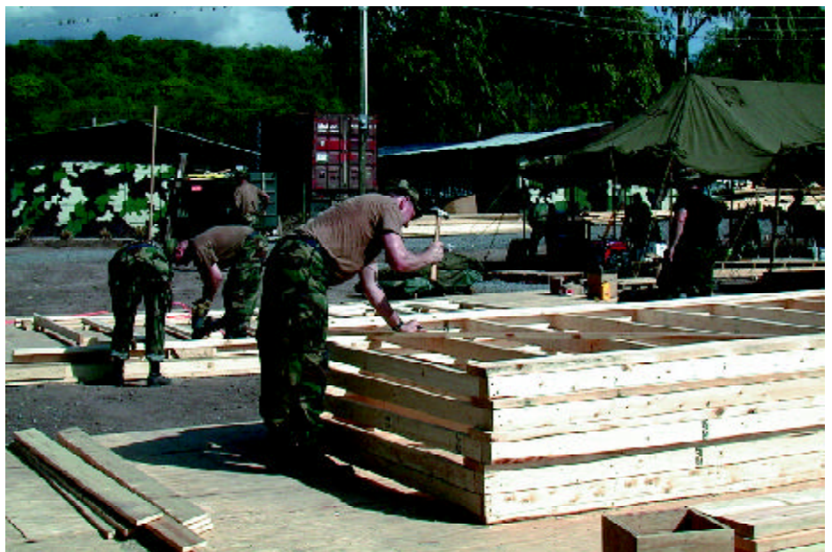
Prime BEEF members construct modular tent floors for transport to a forward base camp. (Photos courtesy 142nd CES)
