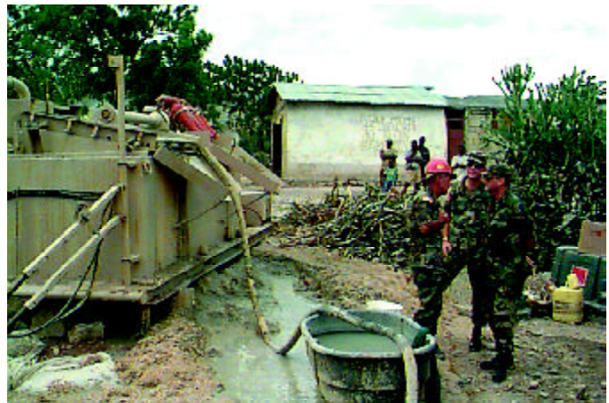
Gen Robbins visited Prime BEEF and RED HORSE construction projects in Haiti. (Photo courtesy HQ ACC)
