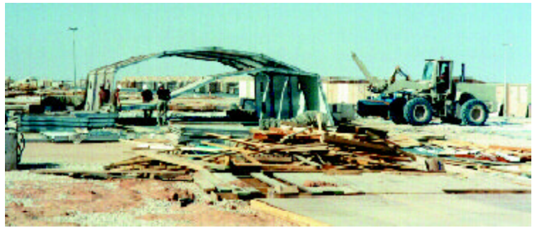
Structures specialists from the 49th Materiel Maintenance Group disassemble a General Purpose Shelter for relocation to the new Friendly Forces Housing Complex at Prince Sultan AB.
