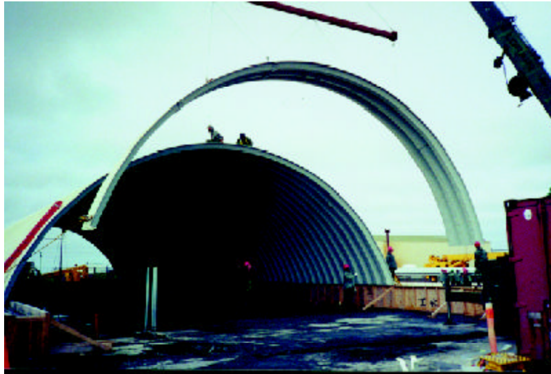
A crane lowers panels into place during RED HORSE construction of a Super K-Span building at Naval Air Station Keflavik, Iceland. (Photo courtesy 203rd RHF)
