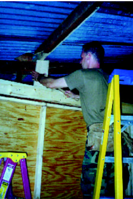
MSgt Chris Bryant, 142nd CES, repairs a termite-damaged roof purlin in the chapel. There was extensive termite damage to the wood structures at the base camp.
