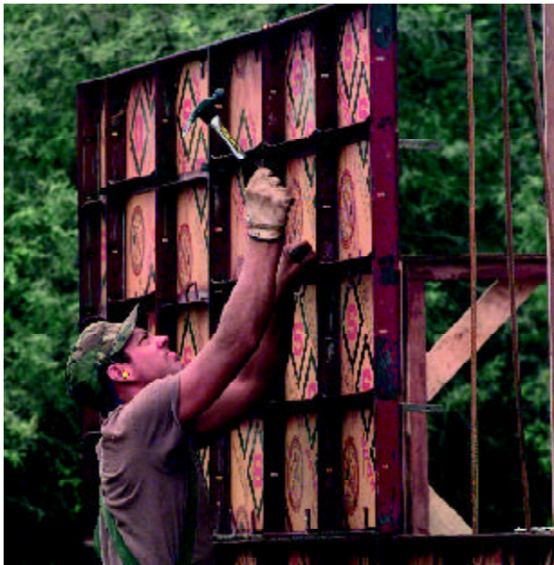
(Right) SSgt John Carter, 819th RHS, hammers a nail into the forms for the wall structure of a two-room school in Camatindi, Bolivia. (Photo by TSgt Katherin D. Bryson)
