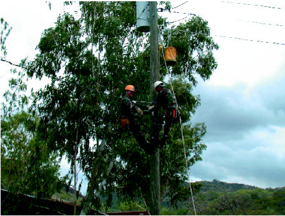
SMSgt Tommy Guerra, 144th CES, and SSgt Rex Rekow, 142nd CES, install a secondary feeder to the billeting area as part of the complete rewiring of the secondary distribution system for the base camp.
