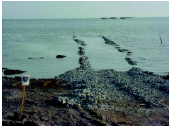
Extreme tide fluctuations allowed only short periods for removing the CBU. Construction of a road, dubbed Red Devil Route 1, into the Yellow Sea allowed quick access to the recovery site during low tide.
