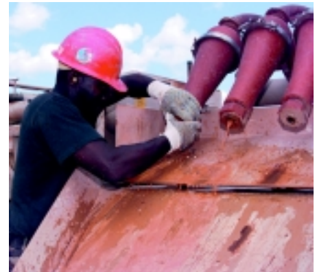
TSgt Willie Daniels, Det 1 307 RHS Power Pro Air Reserve Technician, cleans mud pump spigots which were clogged by sand-sized pebbles during routine mud drilling operations at Pomona, Belize.
