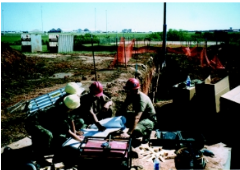
507th CES and 307th RHS members consult project blueprints for a final check prior to encasing the conduit in concrete. Ultimately, laying the power lines underground involved trenching nearly three-quarters of a mile on Tinker AFB. (Photo by SrA Shannon Collins)
