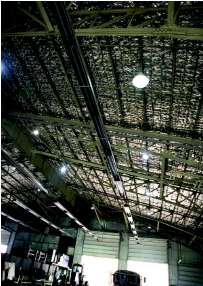
Grand Forks AFB used an ESPC contract to fund base infrastructure improvements such as these gas-fired, infrared heaters. (Photo by TSgt Charles Morris)
