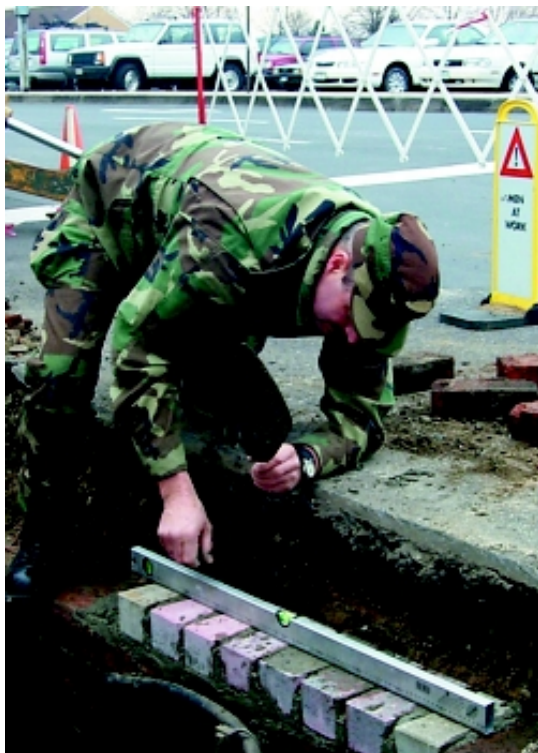
TSgt Gary Simmones, a structures craftsman with the 910th CES, ensures the bricks he is laying are level during a manhole project at Rhein Main AB, Germany, where he was on annual tour. (Photo by TSgt Bryan Ripple)
