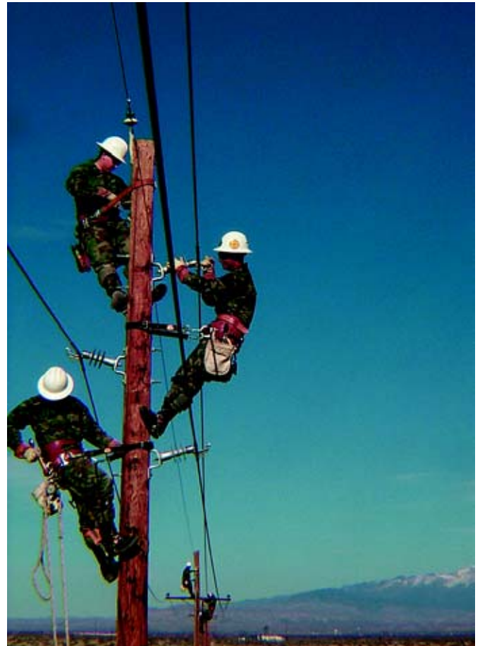
Members of the 49th Civil Engineer Squadron’s Exterior Electric Shop replace outdated utility-pole cross arms at Holloman Air Force Base, N.M. (Photo by A1C Chris Uhles)
