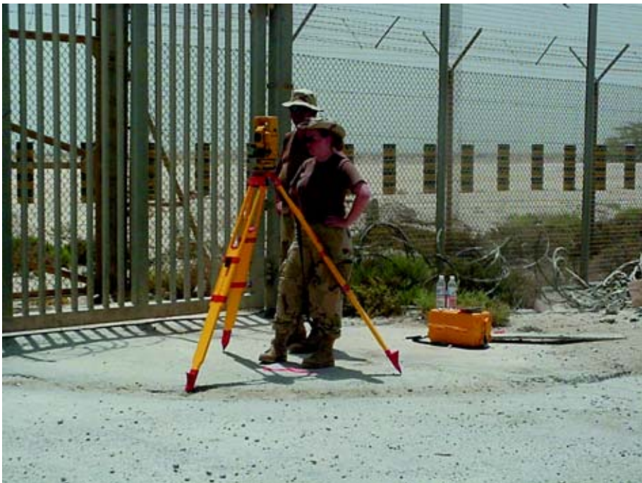
MSgt Terry Smith, 201st RHF, instructs SrA Amanda Rosato, 200th RHS, on the proper construction stake-out of a horizontal curve.
