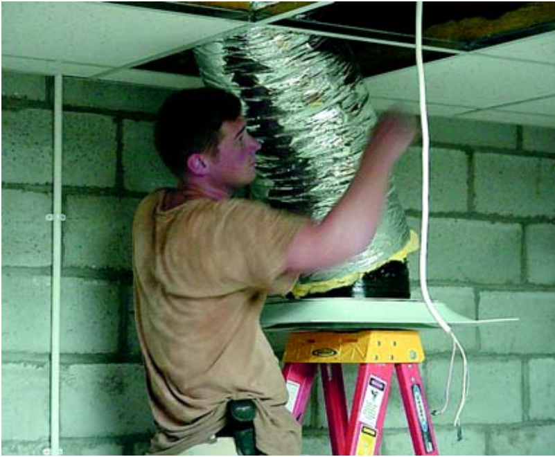
SrA Matthew Bennett, 201st RHF, completes installation of one of the most welcome features in the Base Defense Operations Center facility — air conditioning.
