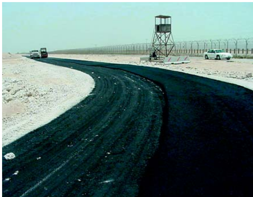
Crosser Boulevard was constructed to redirect vehicle search area traffic at Camp Snoop, Qatar. RED HORSE units completed construction despite 120-degree temperatures. (Photos courtesy 200th/201st RED HORSE)
