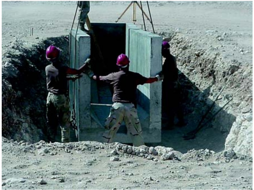
200th/201st RHS personnel place a precast section of the vehicle search pit.
