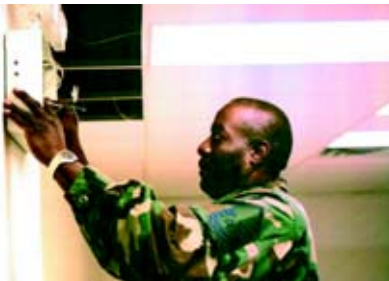
SrA Andre S. Murray (left) and MSgt George W. Anderson (right), both from the 459th CES Electrical/Power Pro Shop, Andrews AFB, perform building renovations for another Andrews tenant, Headquarters Air Force Office of Special Investigations. (Photo courtesy 459th CES)
