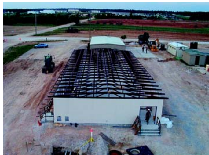
(Top) Construction of an observation tower for monitoring heavy equipment training. (Above) The new classroom facility under construction by the 820th RHS. (Photos by MSgt Ken Willard)
