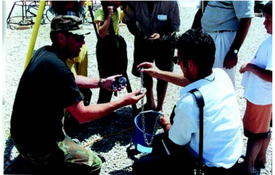
Vermont Air National Guard TSgt Patrick O'Brien (left) helps a Macedonian man assemble a swing set on the playground that civil engineers from Vermont's 158th Fighter Wing helped build for children in Negotino. (Photos by MSgt Bob Haskell)
