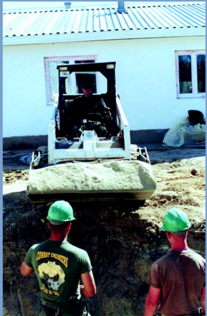
Vermont Air National Guard SSgt Clem Devlin, guided by Marine Corps Reservists, maneuvers a bucket-load of sandy fill over a 15,000-gallon fuel tank beside a medical clinic and community center they helped rebuild in Krivolak, Republic of Macedonia. (Photo by MSgt Bob Haskell)
