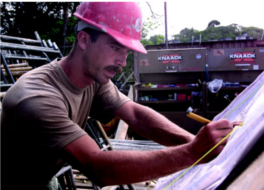
SSgt Daniel Wolfrum, 820th RHS, adjusts the floor plan during construction of the St. Lucia Marine Police barracks. (Photo by SrA Jeanette Copeland)
