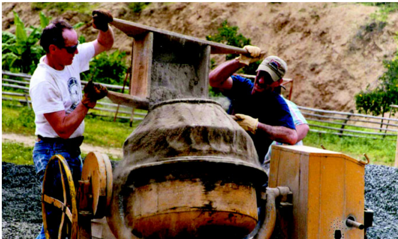
TSgt Todd Peplow and SSgt John Swearingin, both of the 176th CES, pour concrete mix. No concrete mixer trucks were available in the village to aid in the construction of the school.
