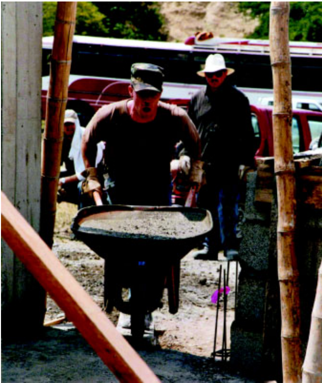
MSgt Charles Sutton, 176th CES, pushes a wheelbarrow full of concrete during the first phase of construction of a new school in a village in Ecuador. (Photos by Maj Donna Prigmore)
