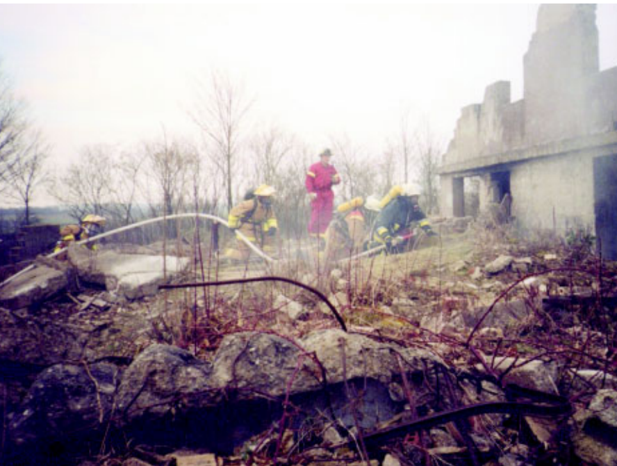
Firefighters advance a fire stream into the basement to begin an interior fire attack and search the basement for trapped victims. (Photos courtesy 469th ABG)
