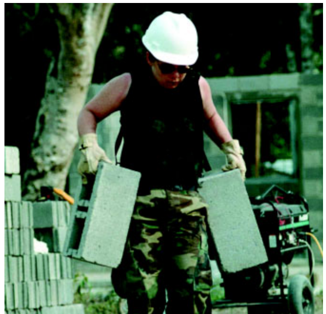
TSgt Peggy Abbott, 908th CES, Maxwell AFB, AL, carries cinder blocks to build restroom facilities for the new school constructed in El Porvenir, Guatemala. (Photo by SrA Shannon Collins)
