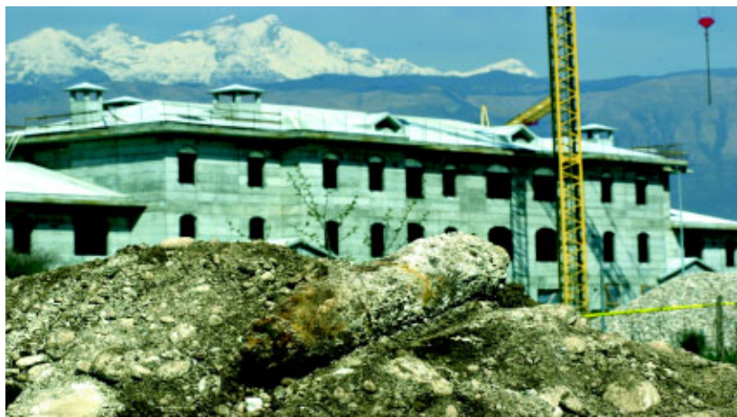
An unexploded AM-30 100-pound, general-purpose bomb dating from World War II rests in the spot that 31st CES members discovered it in April during Aviano 2000 construction. 31st CES explosive ordnance disposal personnel worked with Italian Army explosive ordnance experts to dispose of the bomb. (Photo by SSgt Mitch Fuqua)
