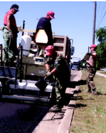
SSgt William Brown, 202nd RHS, clears gutters of excess asphalt during a paving job at Cannon AFB, NM. (Photo by SSgt Paul Cox)
