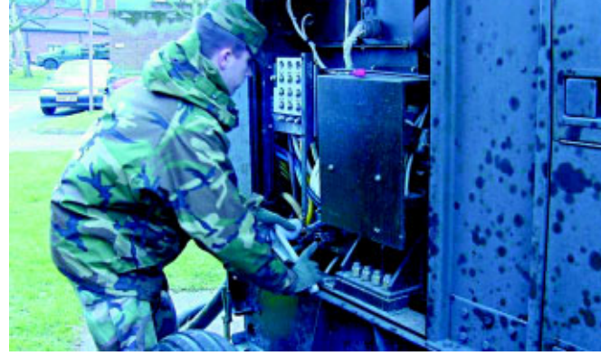
SSgt Karl Danforth connects a load cable to a MEP 7 (mobile electric power) generator. (100th CES photo)
