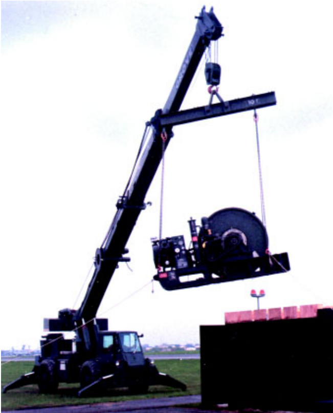
SSgt Andrew Franks, 100th CES Heavy Repair, uses a crane to hoist the old BAK-12 system out. (Photo by SSgt Karl Danforth)
