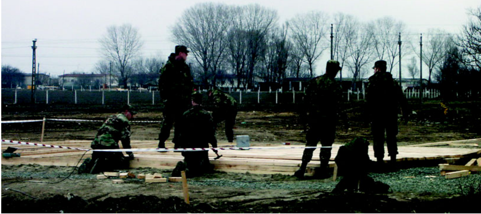
Ramstein AB engineers constructed tent floors to support one of the many missions at Constanta, Romania.
