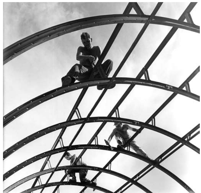
Aviation Engineers construct steel frames for a Quonset Hut roof on Saipan during World War II. (U.S. Air Force photo)
