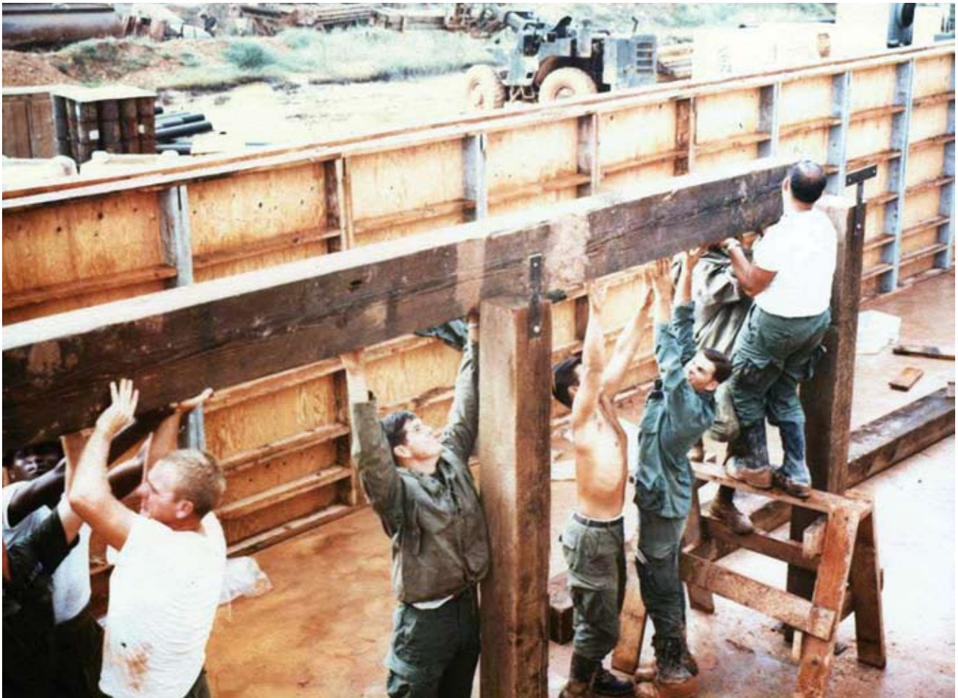
Prime BEEF and RED HORSE engineers proved their worth by building Air Force facilities during the Vietnam War. (U.S. Air Force photo)
