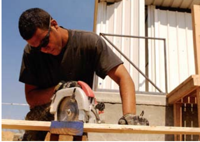
SSgt Justin McRoberts, a structural craftsman from the 820th RHS, Nellis AFB, Nev., cuts stairs for the latrine at the clinic construction site in Buena Vista, Nicaragua. (photo by SSgt Jason Bailey)
