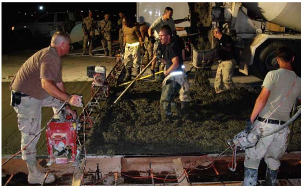
At Balad AB, pouring concrete at night lessens thermal stress on fresh concrete used for runway joint repair. (U.S. Air Force photo)
