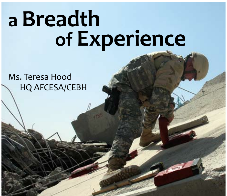
CMSgt Patrick Abbott, 557th ERHS Explosives Demolition Team, sets C4 breaching charges to clear debris from a damaged overpass on MSR Tampa, 20 miles south of BIAP. (photo by TSgt Brandon Lancaster)
