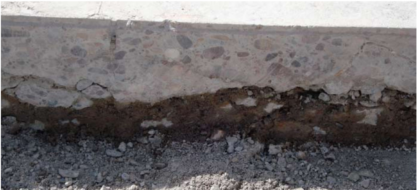
Sulfate attack caused deterioration of the concrete runway. (U.S. Air Force photo)
