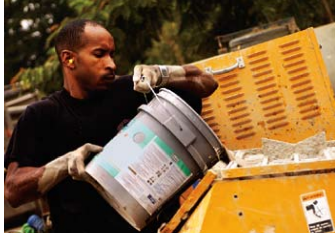
SrA Jean Daniel Colas, 820th RHS, mixes concrete for a pedestal that will hold a dedication plaque at a school being constructed in San Martin De La Calera, Nicaragua. (photo by SSgt Jason Bailey)
