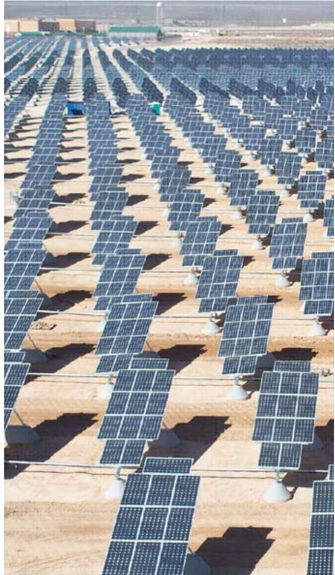
The largest photovoltaic solar power plant in the Americas is a reality at Nellis AFB, supplying 25% of base energy needs. (photo by A1C Nadine Barclay)
