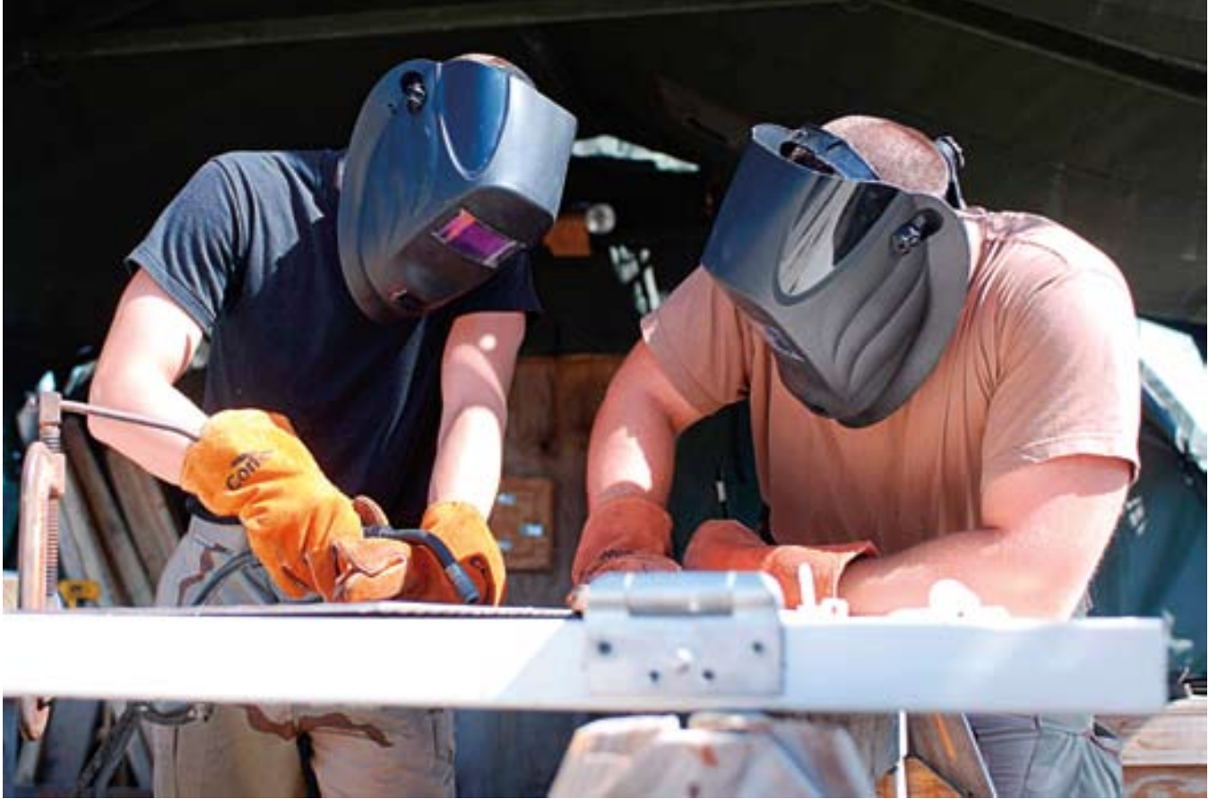
SrA Nick Skinner and SSgt John Heiser weld a detainee cell door at Naval Station Guantanamo Bay. Both are members of the 474th ECES, which was assigned the task of building the Expeditionary Legal Complex. (photo by Army Spc. Shanita K. Simmons)
