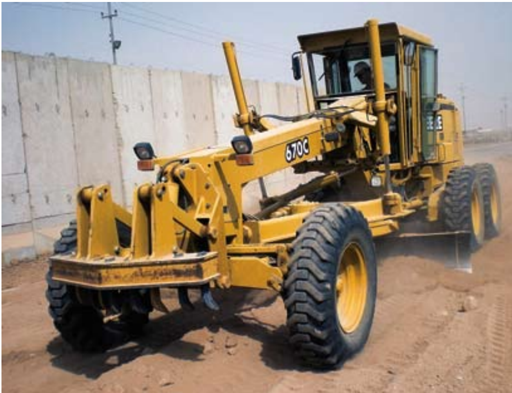
SSgt Stephen Hansen grades an area of dirt where other Dirt Boyz will pour a concrete pad at FOB Caldwell, Iraq. (photo by SSgt Josh Jeffreys)
