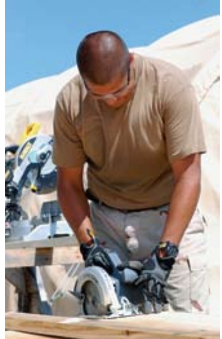
SSgt Alfonso Castro, 474th ECES, cuts out wooden floorboards to prevent flooding in tents at JTF Guantanamo's Camp Justice. (photo by the author)
