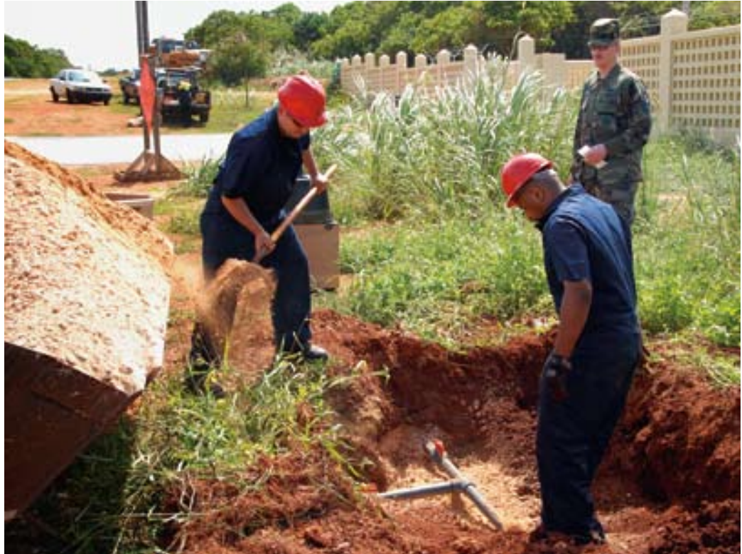
TSgt Jerry Hedstrom looks on as Tgt Todd McGee and TSgt Javier Vigil finish a new pipe and valve installation at the gate of Northwest Field, Guam. (photo by the author)
