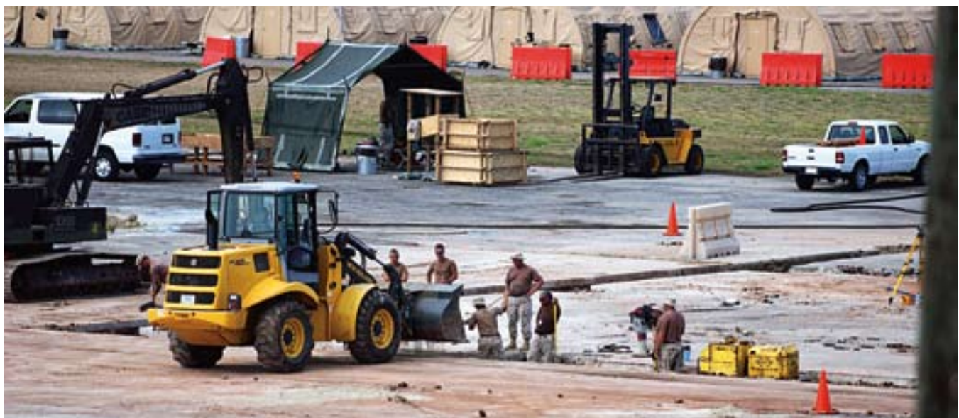
“Dirt Boys” from the 474th ECES prepare to lay a permanent foundation for Naval Station Guantanamo Bay’s new military commissions courtroom. (photo by Army Sgt. Sarah Stannard)
