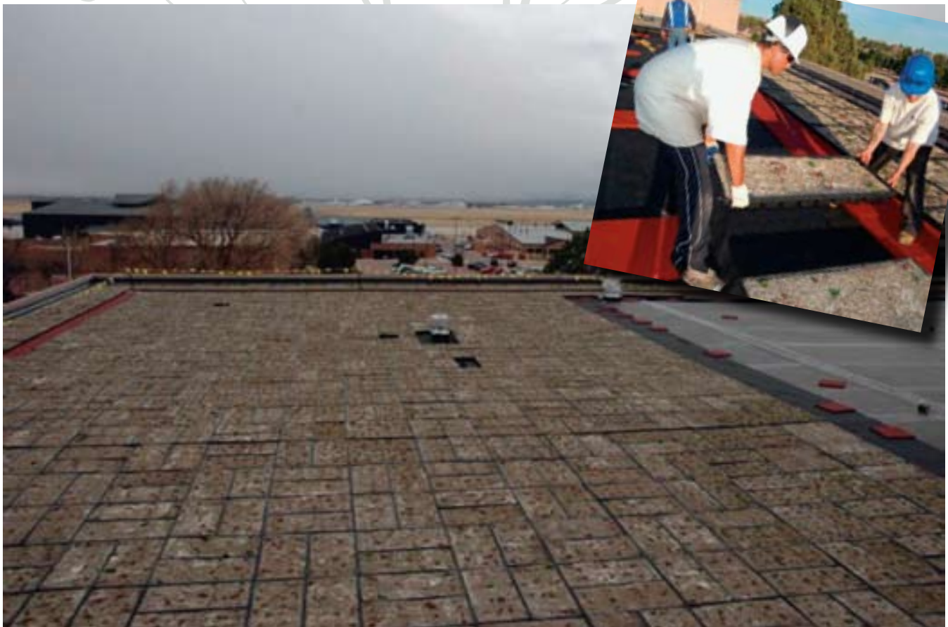
This roof at Peterson AFB will be completely covered in flats of growing media for various types of plants. But first, each one has to be lifted into place by hand. (U.S. Air Force photos)
