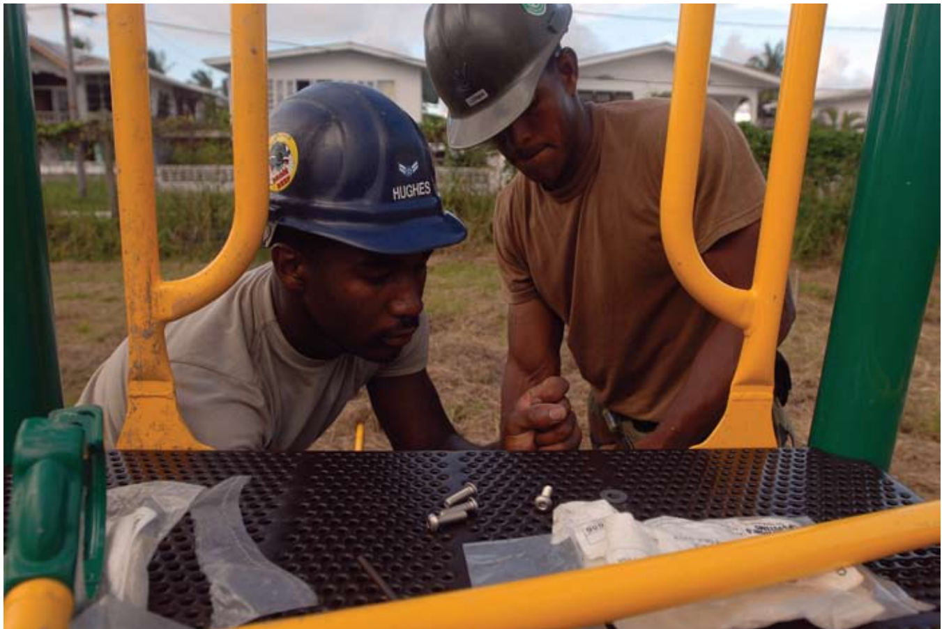
A1C Pasha Hughes, left, of the 5 CES, and Navy Seabee Hugo Lerma work together building a new playground for a local community in Guyana. (U.S. Navy photo by MC2 Gina Wollman)
