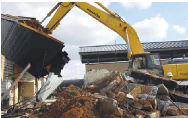
As part of Shaw AFB's demolition efforts, Col Francis Xavier, 20 MSG commander, makes the first blow to a 60-year-old building on the South Carolina base. (SSgt Henry L. Hoegen, Jr.)
